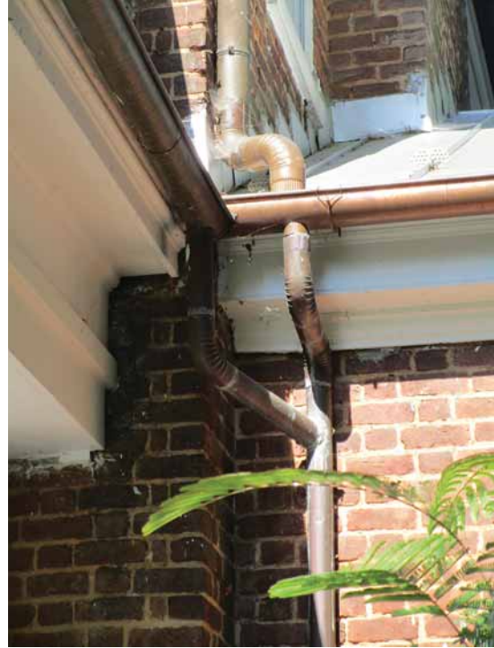
Figure 260. Many of the gutter downspouts on the house follow a circuitous route to the ground. In this location, north of the east porch, three gutters drain into one downspout. JGWA, 2024.
