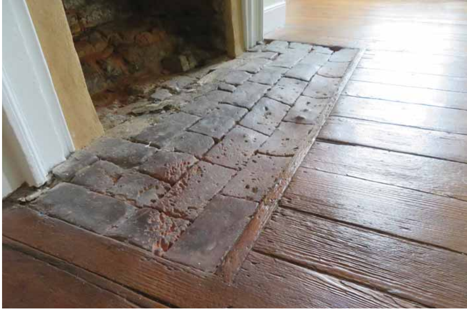
Figure 279. The brick thresholds of each fireplace are worn and the mortar joints eroded, but in the east bedroom (201) this condition is particularly severe. The wood flooring adjacent to the hearths is often similarly worn. JGWA, 2024.
