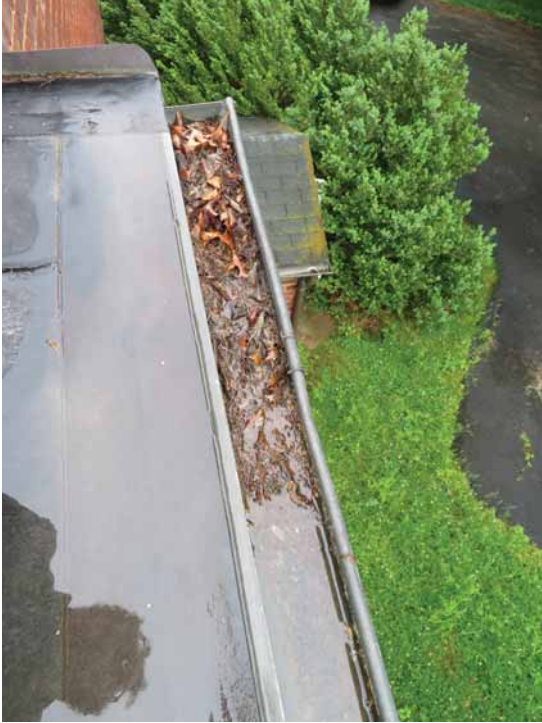
Figure 259. Clogged or nearly clogged gutters exist at all sides of the building. The sheet-metal gutter to the left of this image is intended to prevent water from running down the brick wall below; however there is water damage on the brick below. The asphalt roof on the entrance to the south basement is nearing the end of its service life. JGWA, 2024.
