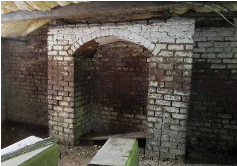
Figure 271. Evidence of rising damp can be seen across the midsection of the hearth support in Room 002 where the limewash has fallen away from the deteriorated face of the brick. There are also deteriorated mortar joints in this section of the wall. JGWA, 2024.
