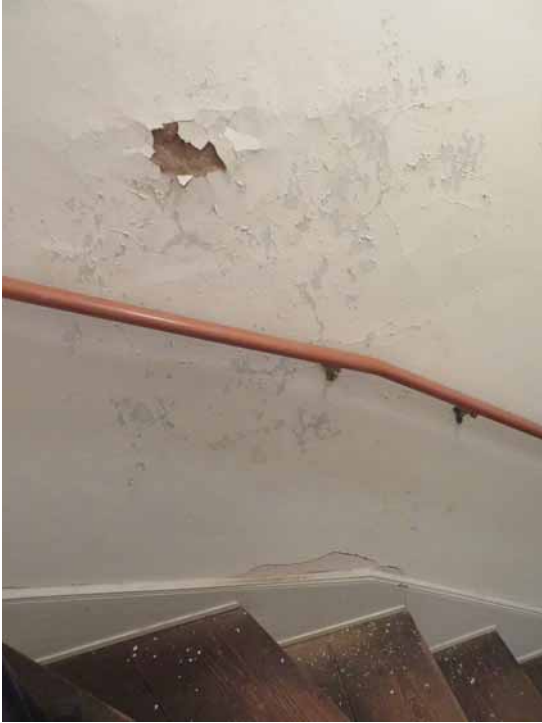
Figure 275. The north wall of the north stair (C101) is in extremely deteriorated condition. This is the result of moisture ingress from the exterior where the north wing and main blocks of the building meet and roof water runs down the face of the exterior wall. JGWA, 2024.
