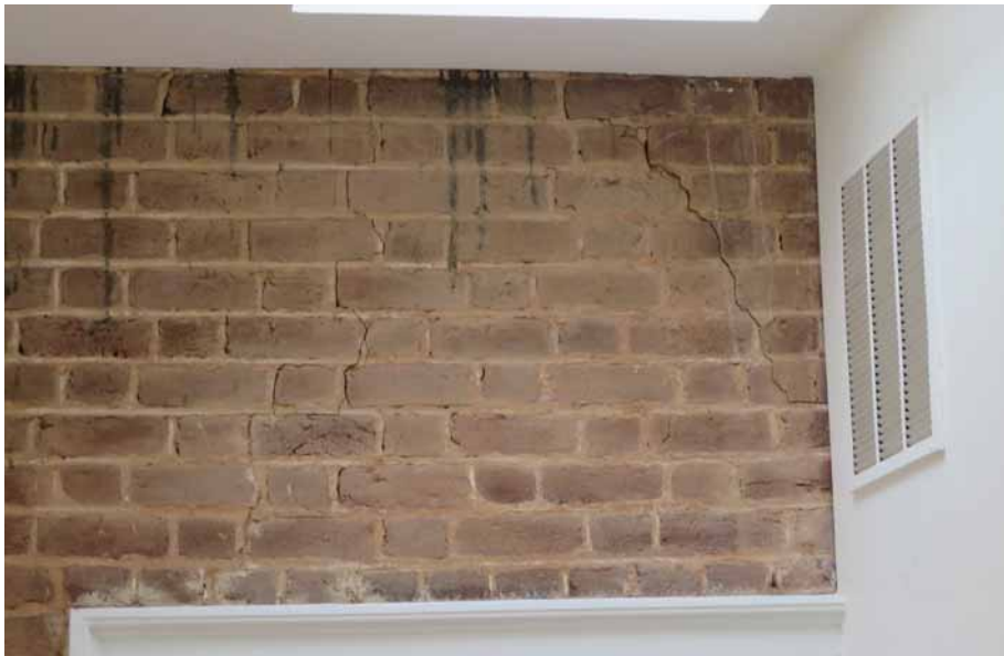
Figure 278. Settlement cracks can be seen in the well-preserved exposed brickwork above two of the doorways in the southwest addition (109). In the image, one of the cracks is over the doorway to the west room (105). JGWA, 2024.
