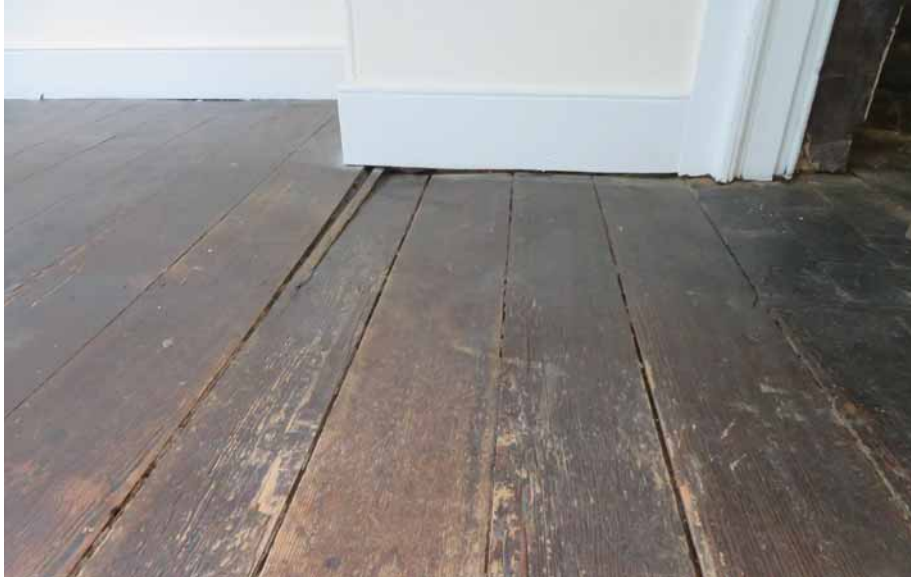
Figure 280. The west end of the floor boards to the south of the fireplace in the west bedroom (205) have dropped out of position. This condition is likely the result of moisture-based deterioration where the roofs above the kitchen and the southwest addition merge. JGWA, 2024.
