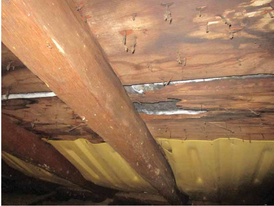
Figure 281. Rotted roof sheathing was left in place in some locations when the roof of the north wing was replaced. In other areas extensive repairs to framing and decking were undertaken. JGWA, 2024.
