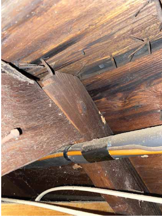
Figure 251. (Left) The rafters meet at mortise-and-tenon joints at the peak of the gable. JGWA, 2024.
