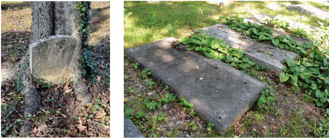
Figure 157. Tree growth has engulfed one of the headstones in the Bramham-Bibb family cemetery (left), while a ground hog has burrowed beneath one of the vaults in the Fife family cemetery (right), threatening the stability and condition of these grave markers. LSHLA, 2024.
