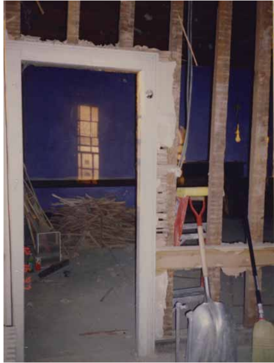
Figure 248. The second-floor bathroom (T206) during the 1997-1998 work, after the lath and plaster were removed. Courtesy of Nancy O'Brien.
