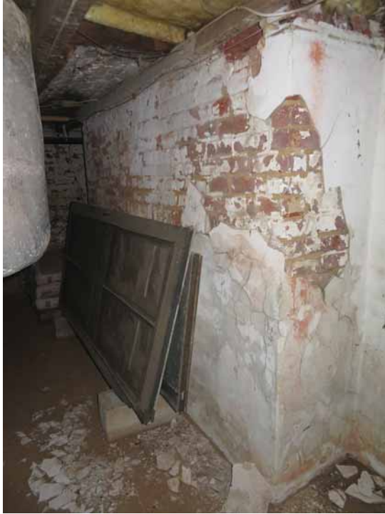
Figure 273. (Left) The cementitious render that was applied to much of the brick wall surface in the south basement (001) has fallen away in sheets where it has trapped rising moisture. In these locations, the brick is more damaged than in areas where only limewash was applied to the brick surfaces. JGWA, 2024.
