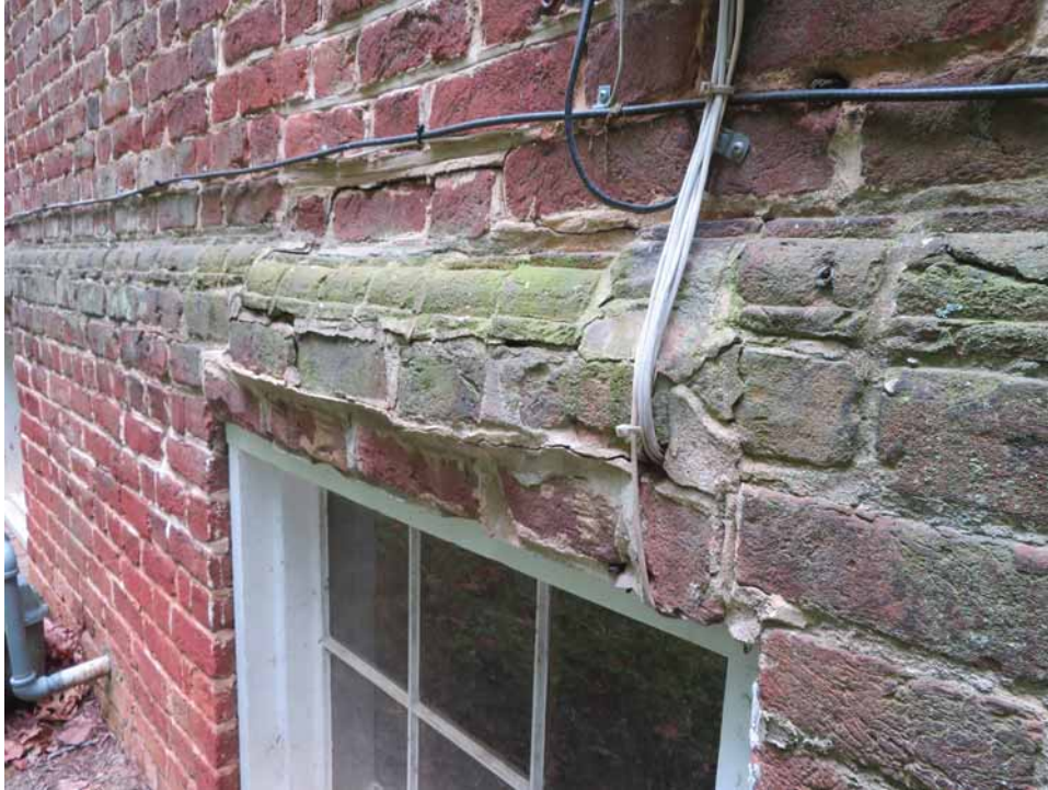
Figure 264. (Below) In many instances, there is displacement of the bricks where the molded brick water table passes over the basement windows. This condition is most advanced at the westernmost window on the north side of the main block of the house. JGWA, 2024.
