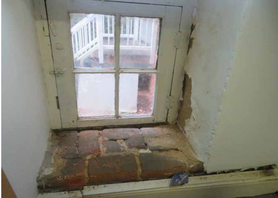
Figure 277. The plaster failure on the east side of the small window in the storage room under the stairs (106) is the result of moisture ingress. In this location, overflow from the roof has caused an area of staining on the exterior face of the wall and related damage on the interior. JGWA, 2024.
