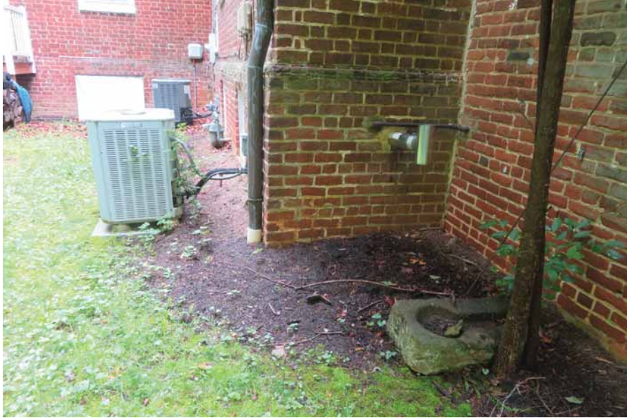
Figure 272. The north side of the central block of the house is a repository for numerous pieces of mechanical, electrical, and telecommunications equipment. It is also the exit point for the direct vent of Oak Lawn's boiler. JGWA, 2024.
