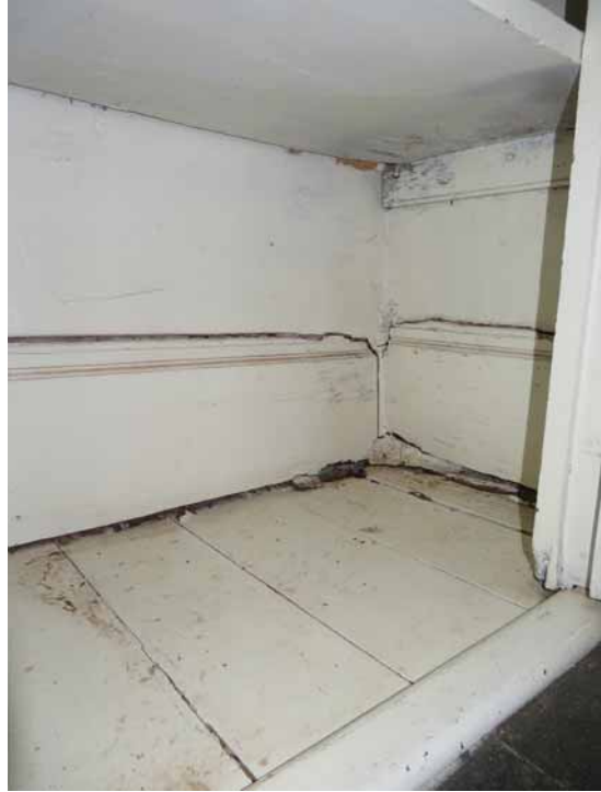
Figure 276. The floorboards under the built-in cupboard in the northwest corner of the west room (105) have dropped out of position, as has the baseboard above. This condition is a result of moisture-based deterioration adjacent to a failed roof leader. JGWA, 2024.
