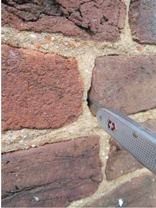
Figure 263. (Left) Head joints, the vertical joints at the small ends of individual bricks, are often not filled as well as the bed joints below each brick during construction. When the surface joint in these locations fails, a void often exists behind the surface. JGWA, 2024.
