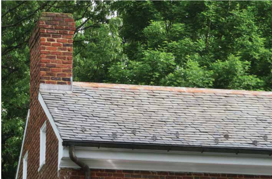
Figure 255. Slate shingles cover the central section of the roof, which shows signs of its age through missing, broken, and displaced slate. Regular maintenance has countered some of the age-related deterioration. JGWA, 2024.
