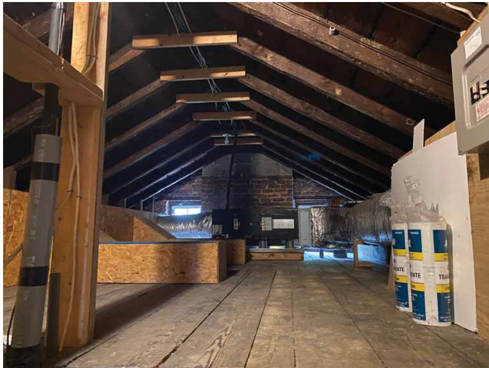
Figure 250. The central attic (301), looking east (upper image) and west (lower image). JGWA, 2024.
