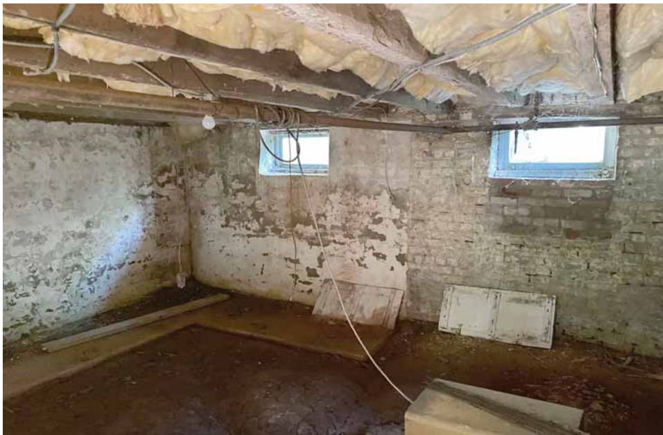
Figure 211. The north basement (002), looking south (upper image) towards the arched support for the fireplace above; and northeast (lower image). Note the brick infill below the windows, indicating their original size. JGWA, 2024.
