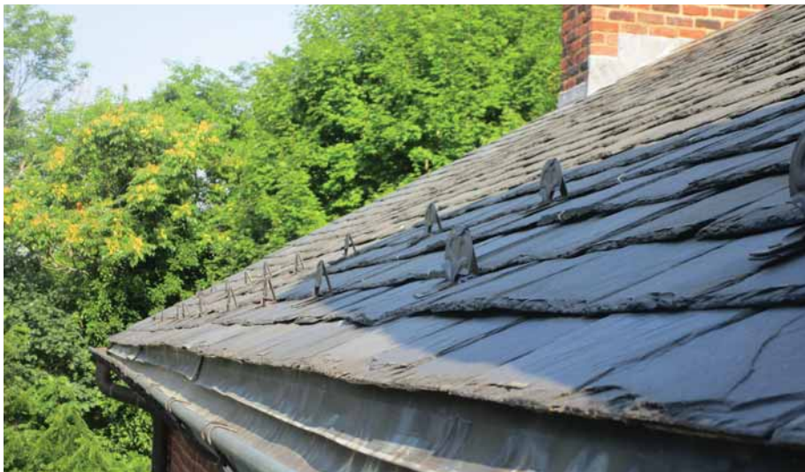
Figure 256. Roof accessories, such as snowguards, flashings, and hung quarter-round gutter are generally in sound condition. Copper hooks used to secure replacement slates can be seen in numerous locations. JGWA, 2024.
