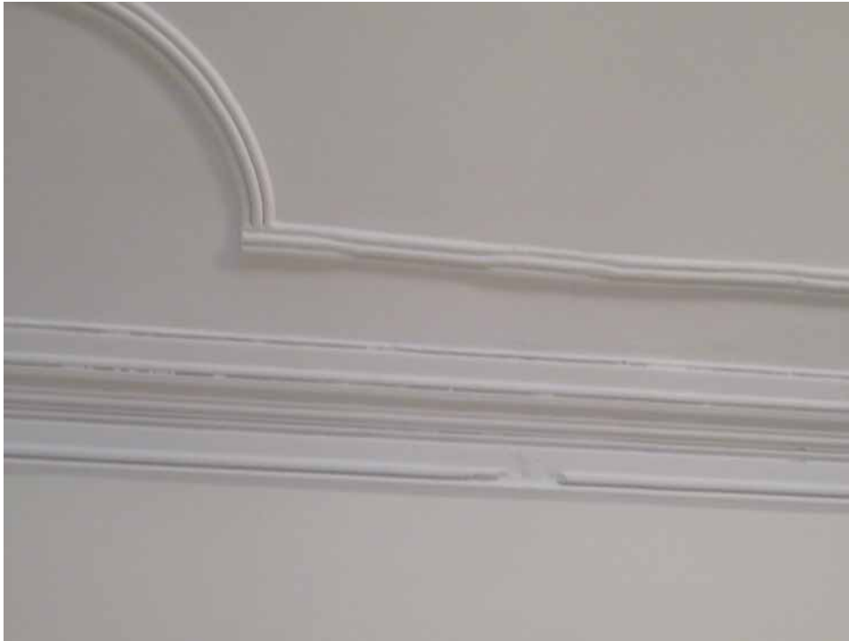
Figure 274. (Below) The plaster ceiling in the entrance hall (101) has been renewed and repaired on numerous occasions. Buildup of paint coatings has obscured some of the details and shadow lines. In some areas cracking of the plaster has resulted from movement and uneven support. JGWA, 2024.
