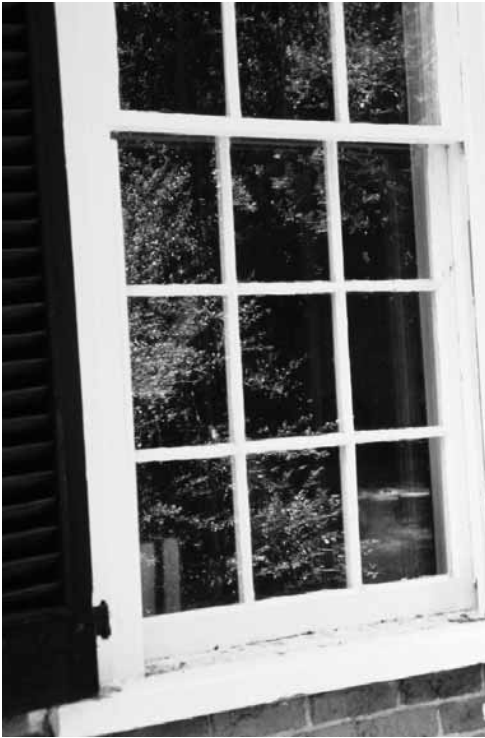
Figure 58. 13 West Range, University of Virginia, Charlottesville, Virginia: detail of window sash, taken by Murray Howard in June, 1998, and noted as prototype for window replacements throughout Grounds.
