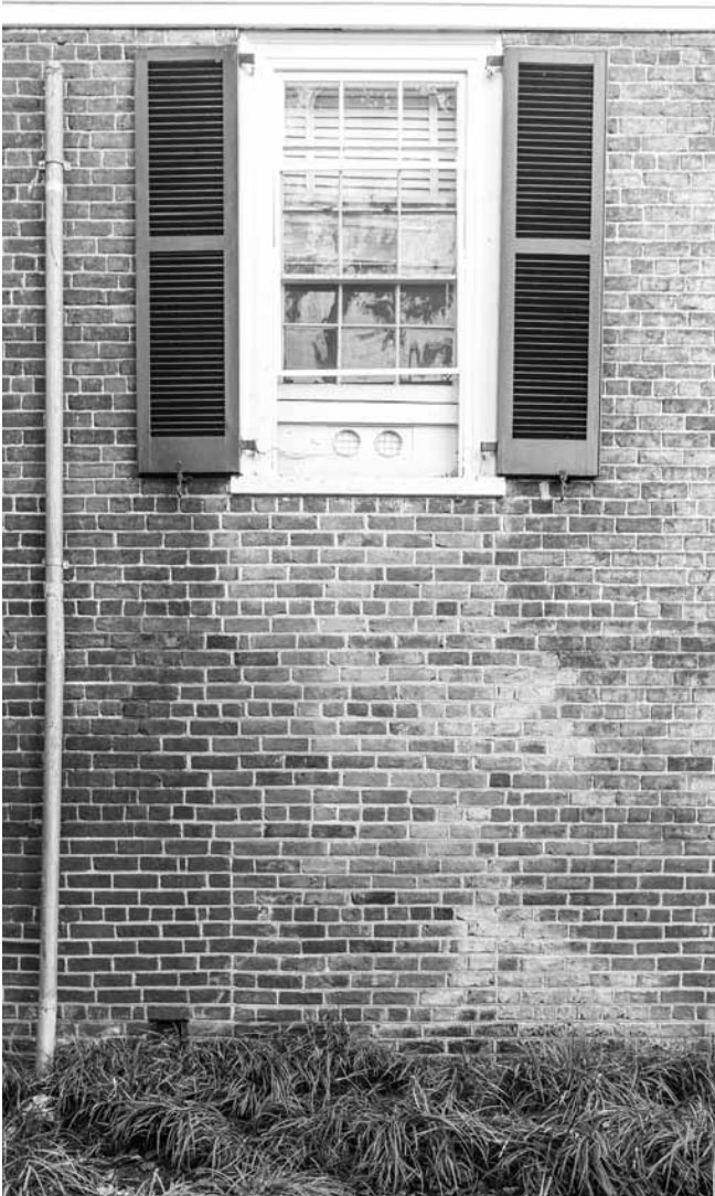
Figure 170. University of Virginia, Charlottesville, Virginia: rear of 48 East Range, with blocked opening at cellar and rebuilt masonry below formerly lowered window, since raised back to original position.
