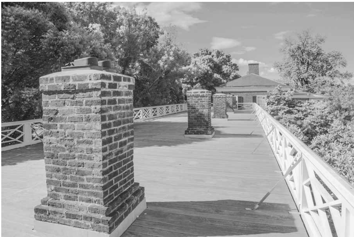
Figure 46. University of Virginia, Charlottesville, Virginia, 35-51 West Lawn roof as restored, looking towards Pavilion IX.
