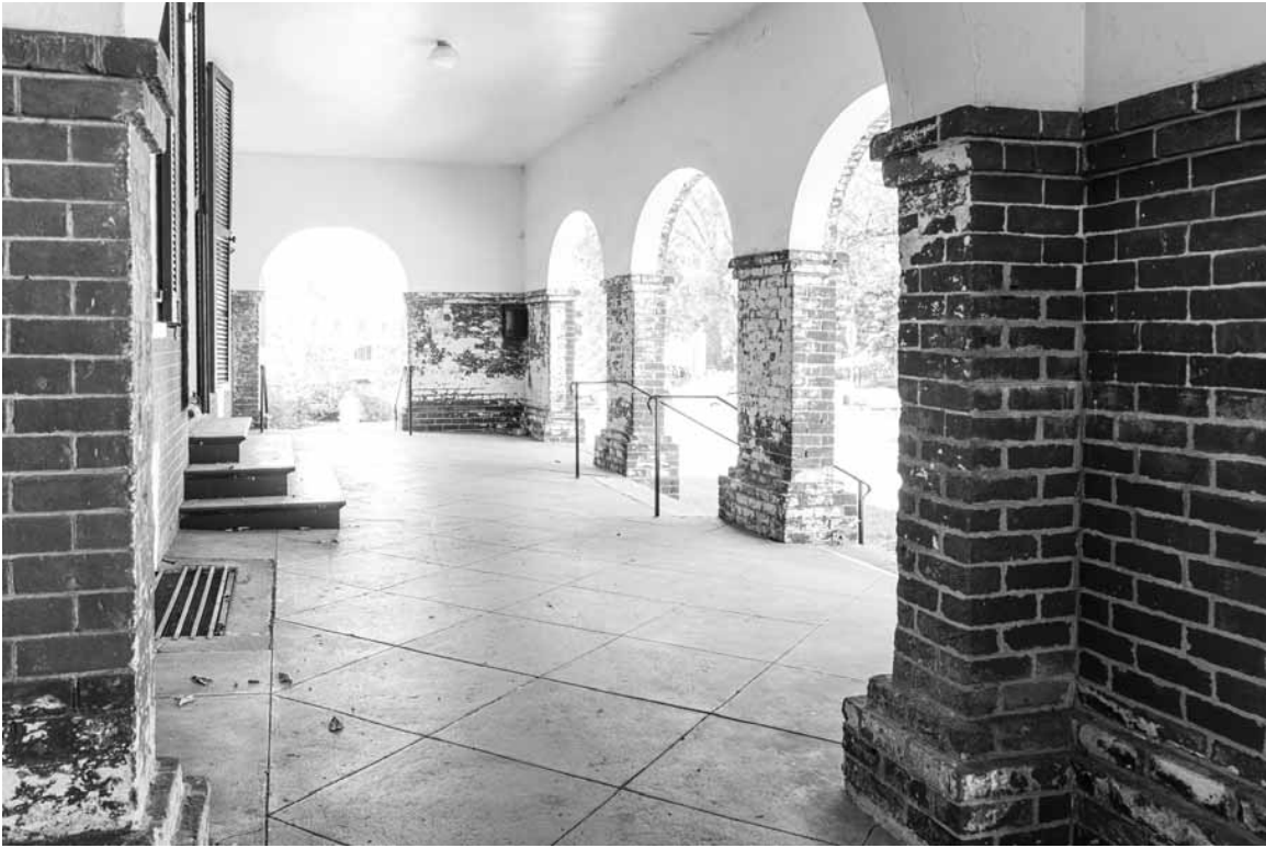
Figure 107. University of Virginia, Charlottesville, Virginia: Arcade at Hotel E, showing remnants of white wash and red wash on inside of arcade and granolithic paving.
