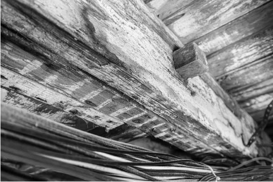
Figure 165. University of Virginia, Charlottesville, Virginia: 36 East Lawn cellar at hearth bed showing doubled joist with through-tenon for hearth timmer and lath stains on underside of joists for plaster ceiling.
