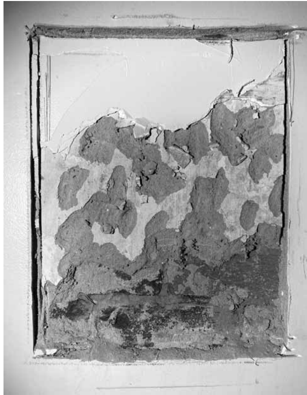
Figure 97. Unidentified University of Virginia Lawn room, Charlottesville, Virginia: detail of plaster repair showing layers of modern skim coats over original brown coat on masonry with original finish coat.
