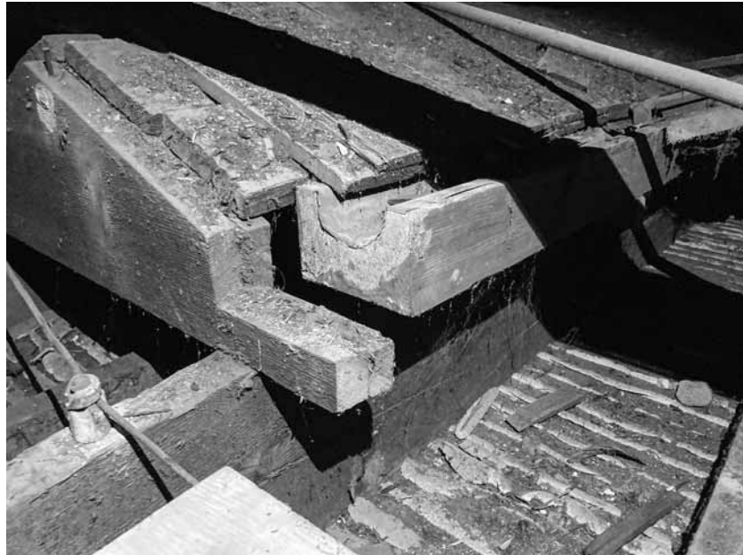
Figure 84. University of Virginia, Charlottesville, Virginia: attic of West Range 5-15 student rooms, showing gutter and doubled serrated lath at center of serrated roof. Note also lath and plaster ceiling below.
