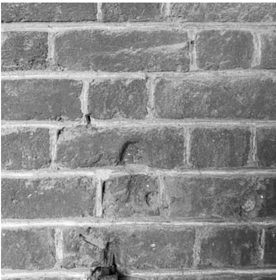
Figure 110. University of Virginia, Charlottesville, Virginia, 13 West Range, detail of brickwork and mortar with painted pointing.
