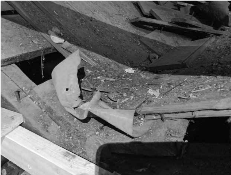
Figure 81. University of Virginia, Charlottesville, Virginia: attic above 23-27 West Range student rooms, detail of tin-lined gutter in serrated roof.
