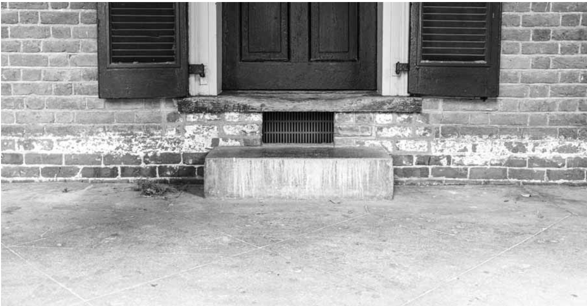
Figure 108. University of Virginia, Charlottesville, Virginia, 10 East Range, showing vent below door sill and re-set bricks to raise floor, whitewash remnants at base of wall, and granolithic paving.
