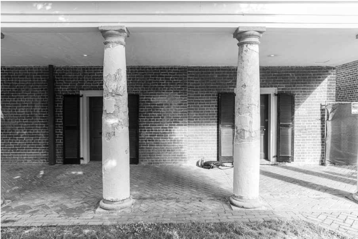
Figure 140. University of Virginia, Charlottesville, Virginia, 21-23 West Lawn, showing break in masonry and rise in level of paving from 23 (at right) to 21 (at left).
