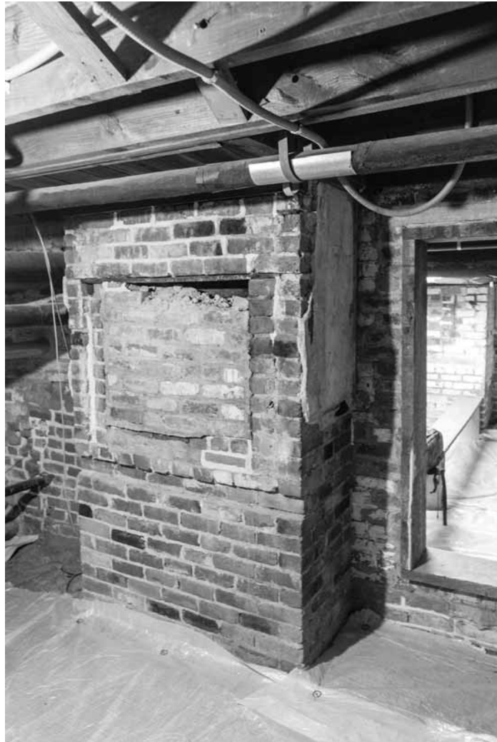
Figure 169. University of Virginia, Charlottesville, Virginia: cellar of 48 East Lawn, looking back towards 46 cellar, showing fireplace and plaster for room above, both installed when floor was lowered for John B. Minor in 1876.
