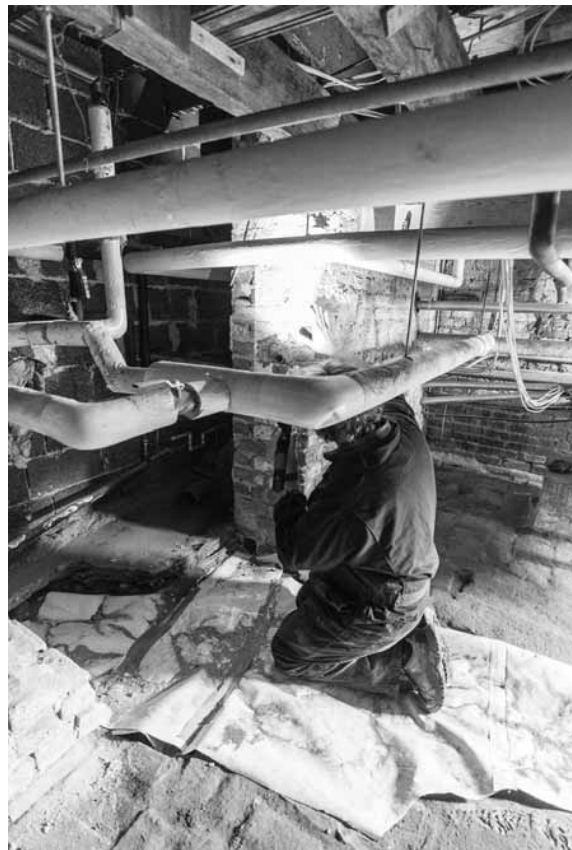
Figure 181. University of Virginia, Charlottesville, Virginia: 24 East Range, cellar, with Eric Gradoia inspecting remnant of masonry jamb in north wall, at opening to cellar of Hotel D. Note pocket at base of wall, paint edge, and flat mortar joints at left side of brick jamb, all showing location of early wood door jamb.
