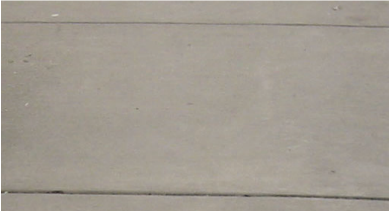
Poured concrete with Canvas colorant by Soloman, joint sealant Sikaflex capital tan
