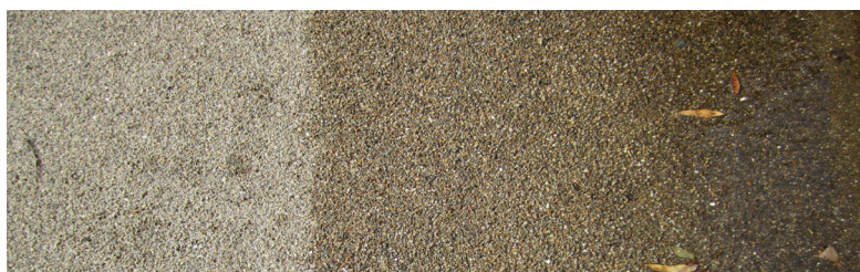
Addastone Resin Bounded Surface System. Above picture taken after rain in Poe Alley.
