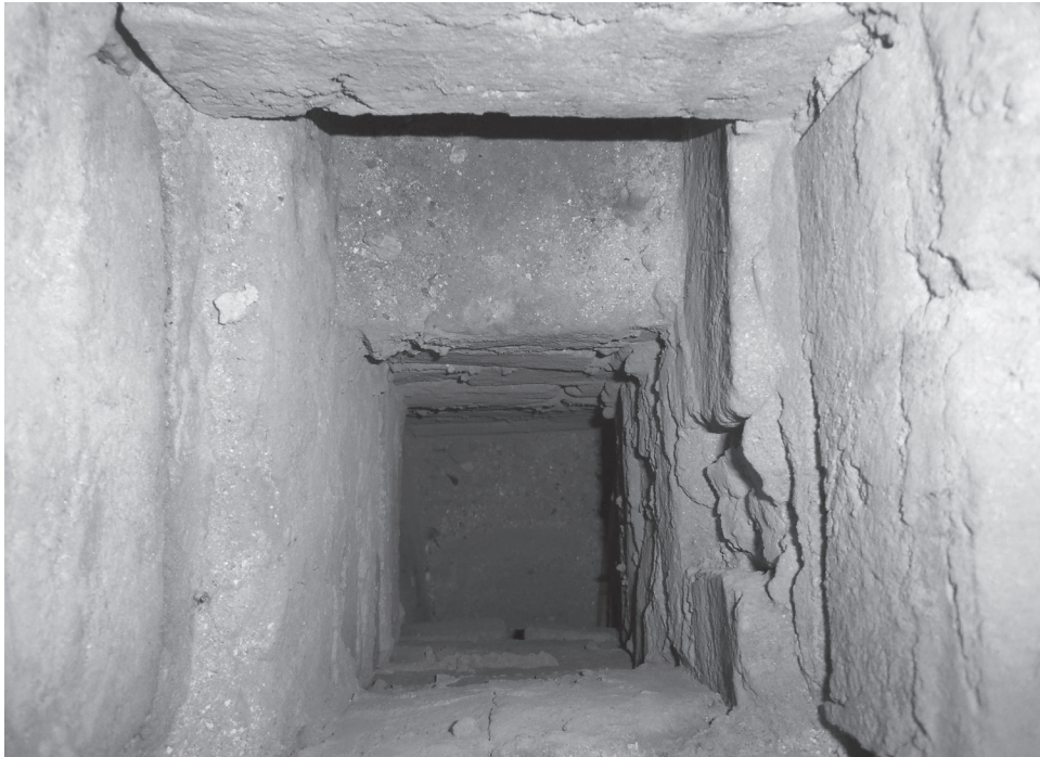
Figure 51. East intermediate station with shelf (upper image); and looking down through the station (lower image). [JGWA, 2014]
