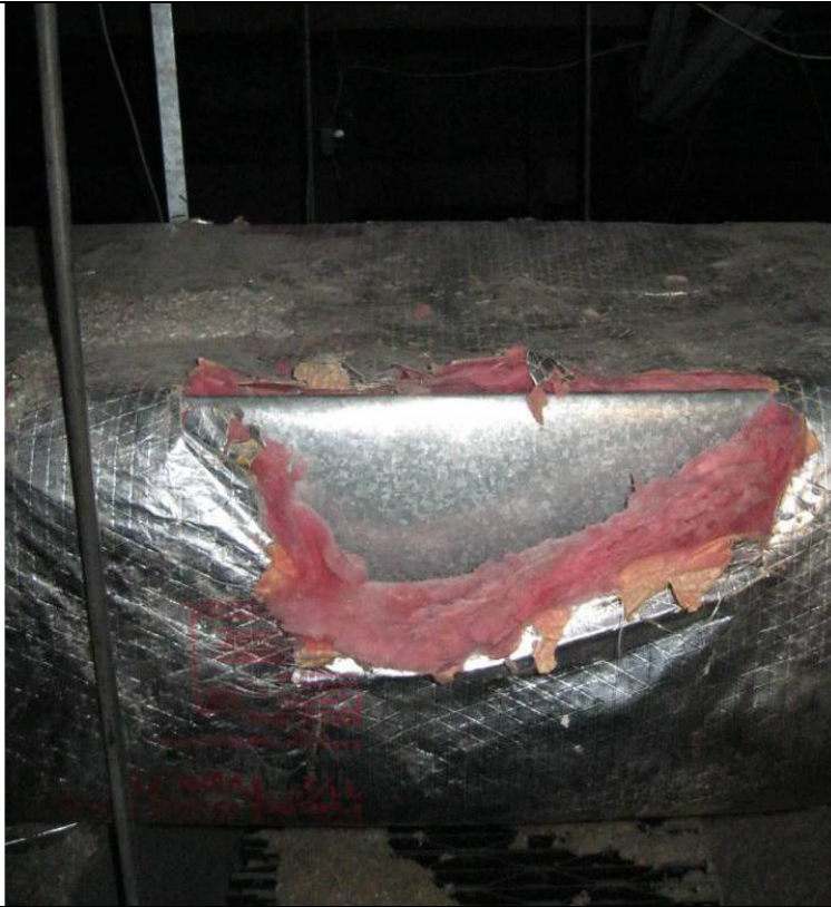
Figure 1.2.4.2-4: Damaged insulation on ductwork in attic. Photograph by T. Newbold, December 2012.
