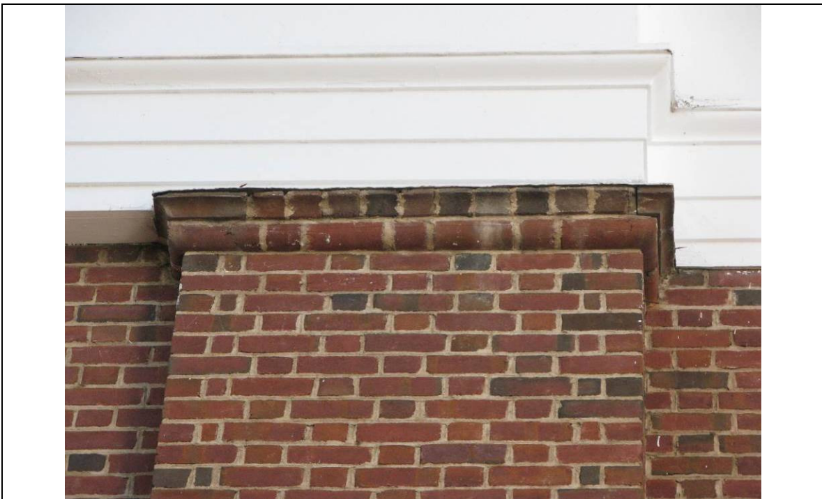
Figure 1.2.3-4: Degraded pointing and rough flashing, typical at pilaster heads. Photograph by John Milner Architects, November 2012.
