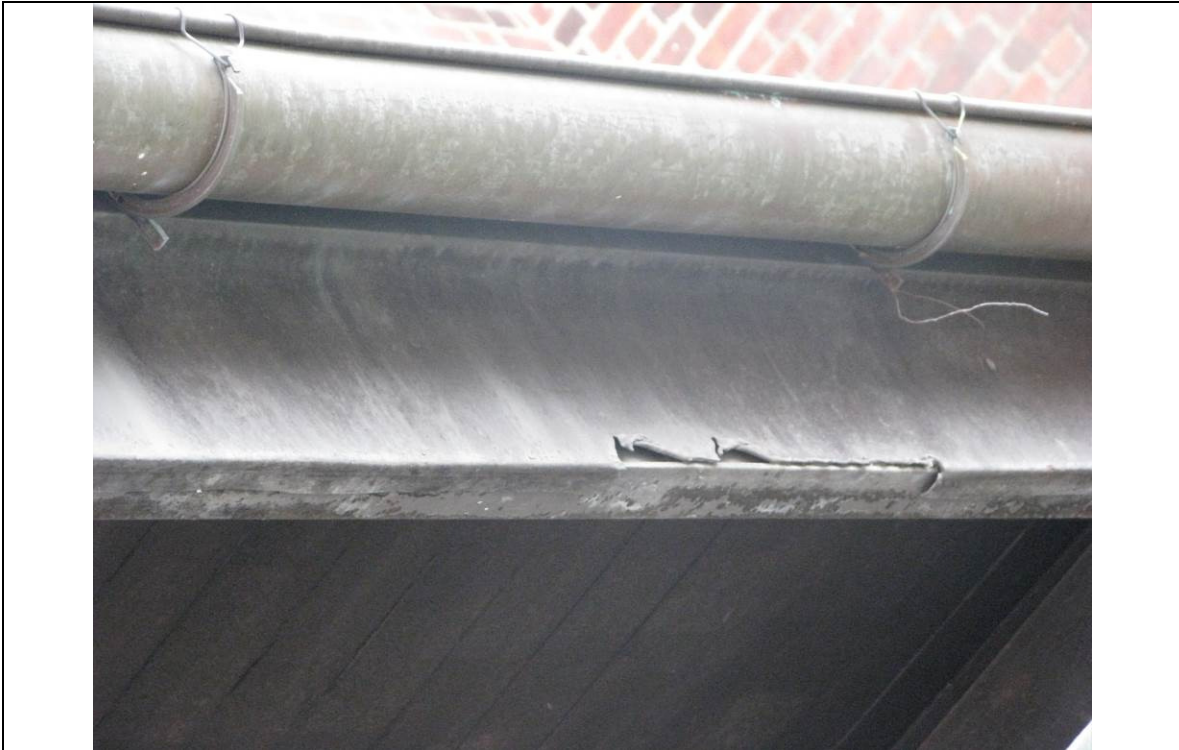
Figure 1.2.3-28: Damaged metal fascia at West canopy. Photograph by John Milner Architects, November 2012.
