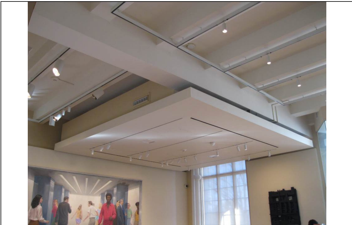
Figure 1.2.4.2-5: Enclosure concealing AHU-4 (typical for AHU-5). Photograph by T. Newbold, December 2012.
