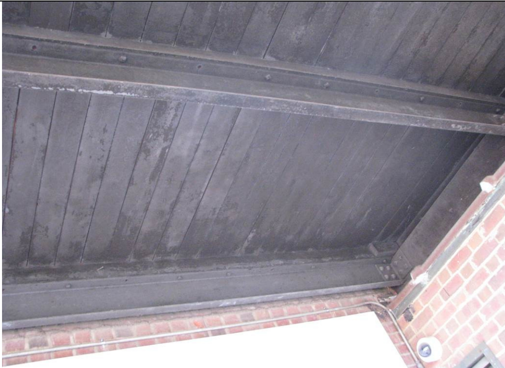
Figure 1.2.3-29: Degraded paint at underside of West canopy. Photograph by John Milner Architects, November 2012.
