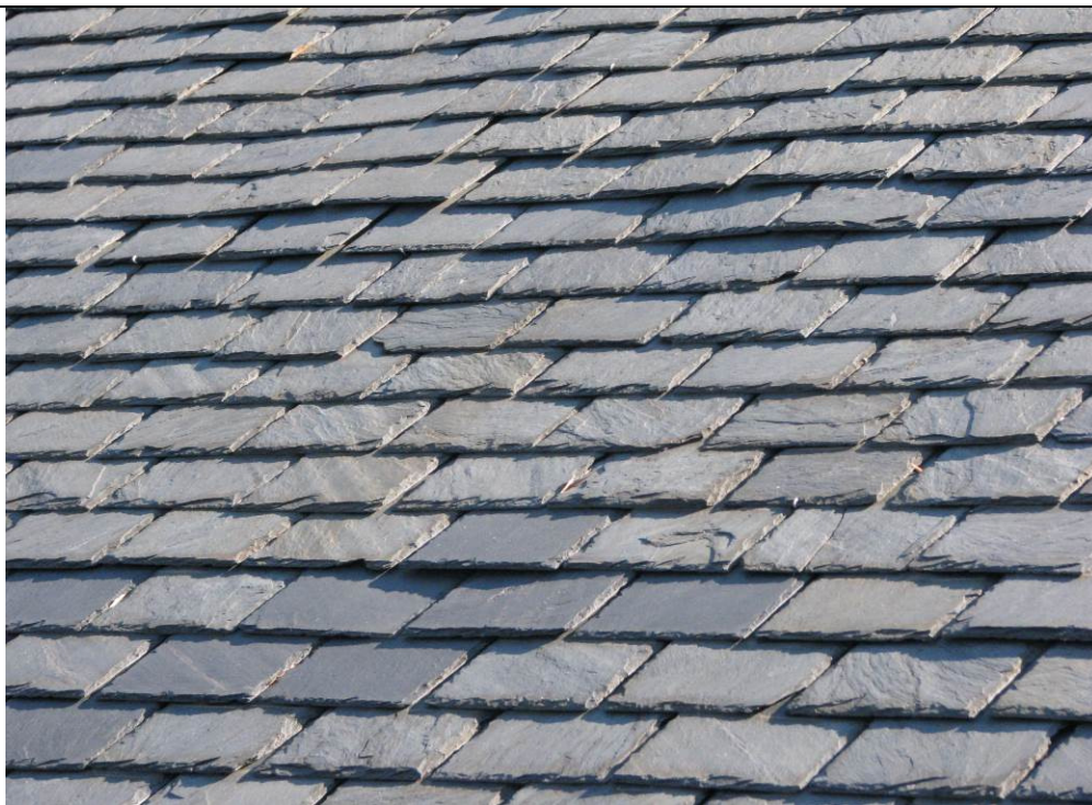
Figure 1.2.3-21: Slates susceptible to breakage at roof undulations. Poorly matched patch in foreground. Photograph by John Milner Architects, November 2012.
