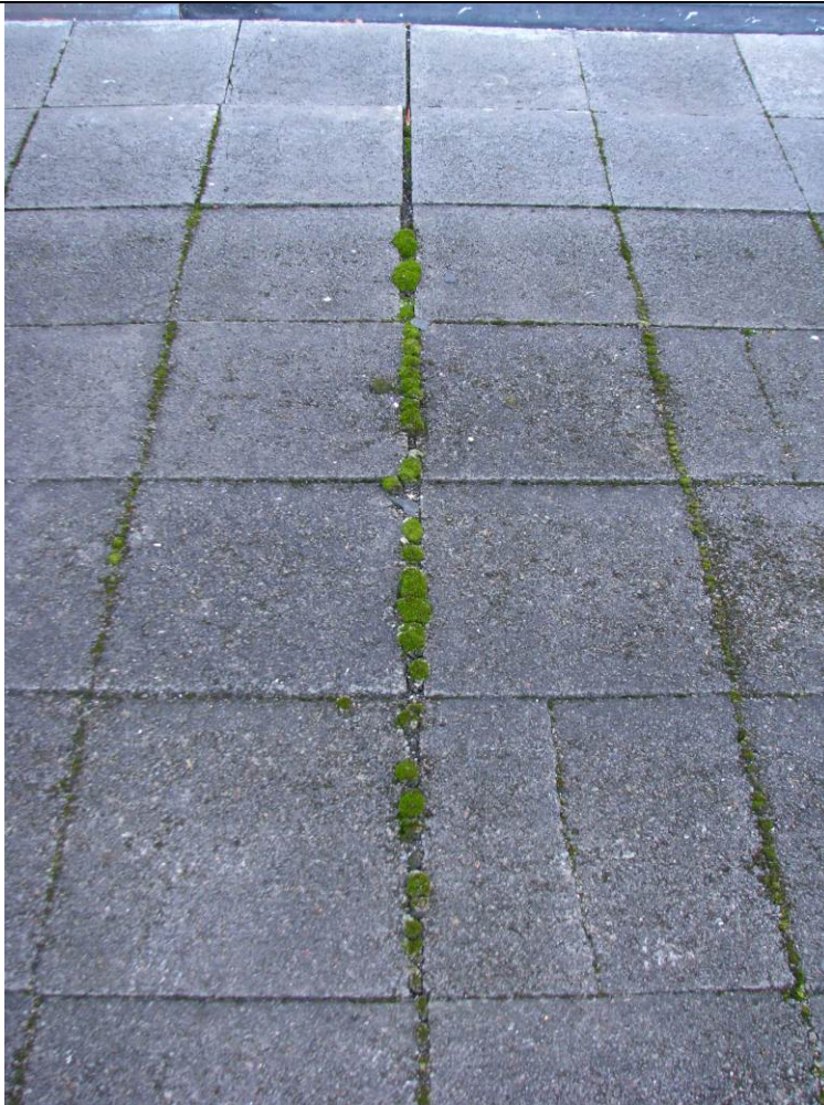
Figure 1.2.3-24: Biological growth at West Terrace pavement. Photograph by John Milner Architects, November 2012.
