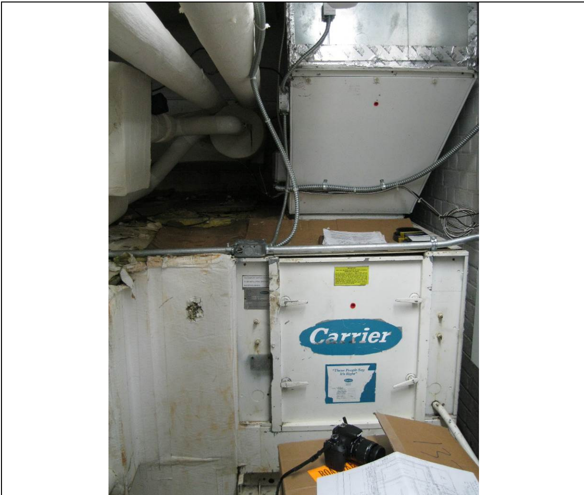
Figure 1.2.4.2-3: Air handler AHU-1. Photograph by T. Newbold, December 2012.
