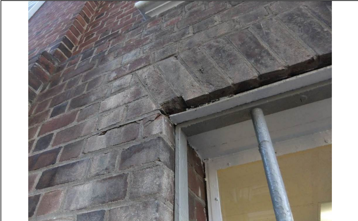
Figure 1.2.4.1-20: Deterioration of brick flat (jack) arch due to rust jacking of supporting steel lintels along North elevation. Photograph by Robert Silman Associates, November 2012.
