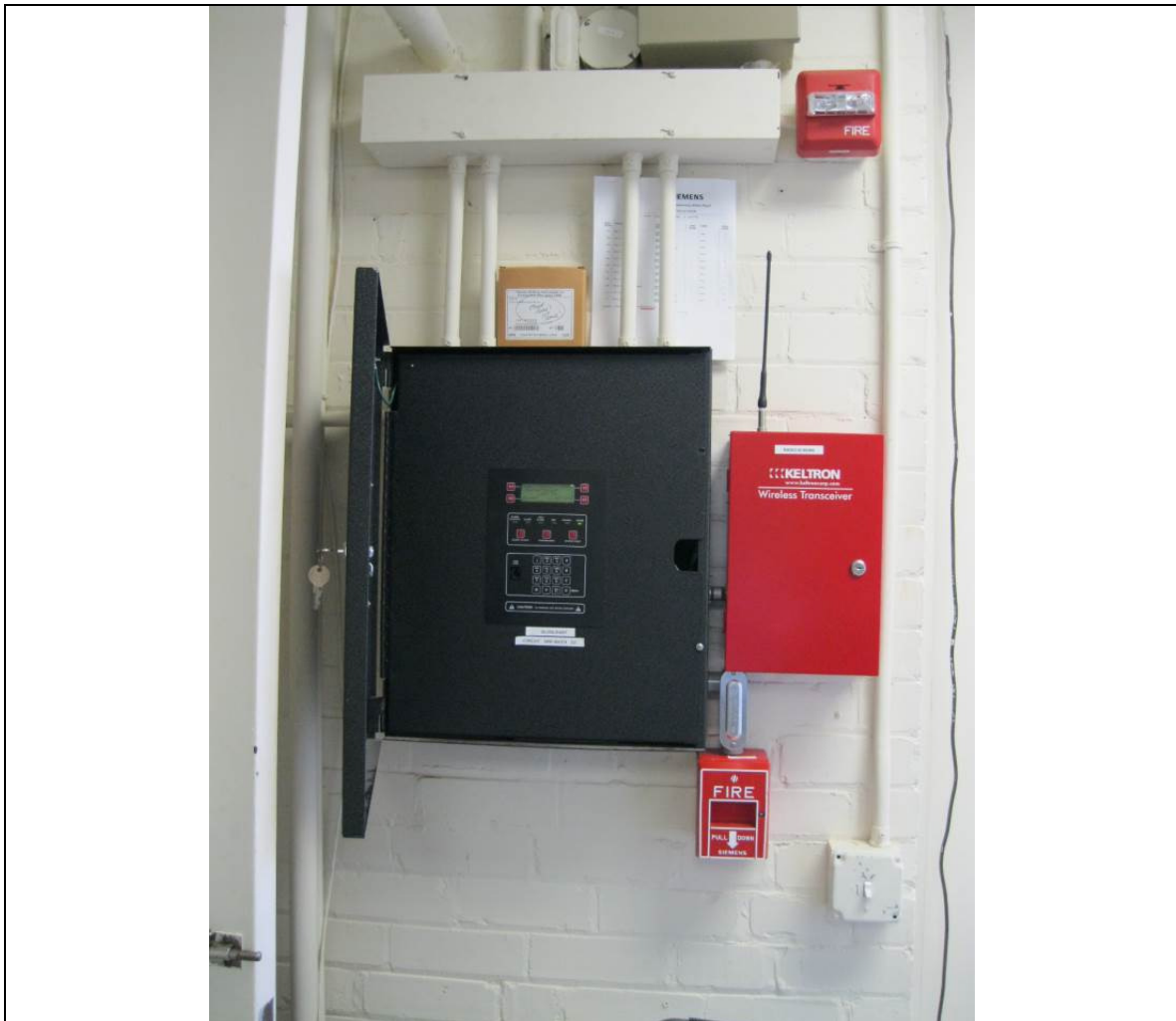
Figure 1.2.4.2-13: Fire-alarm control panel adjacent to lower-level entrance. Photograph by T. Newbold, December 2012.
