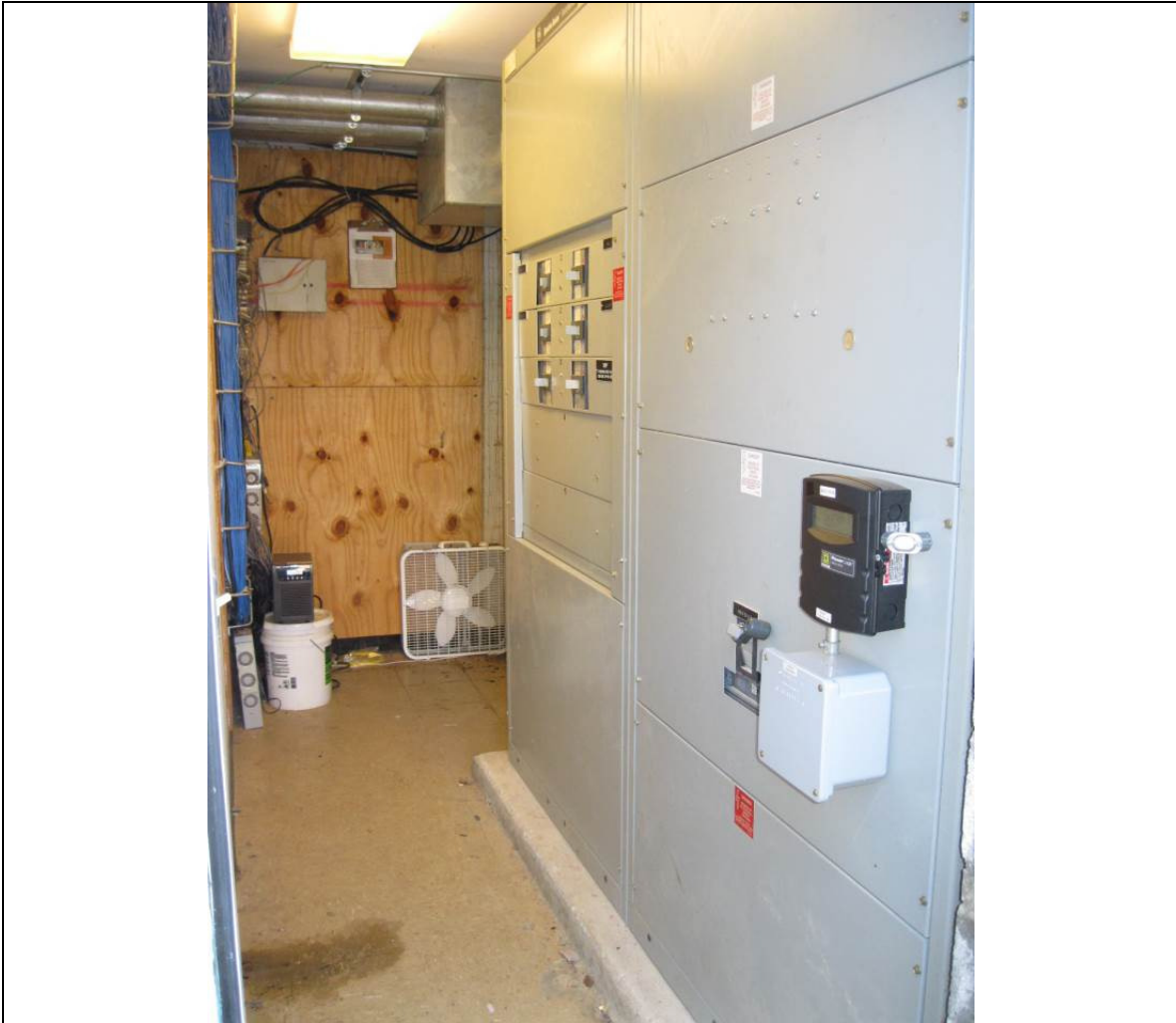
Figure 1.2.4.2-11: Main distribution panel in Annex. Photograph by T. Newbold, December 2012.
