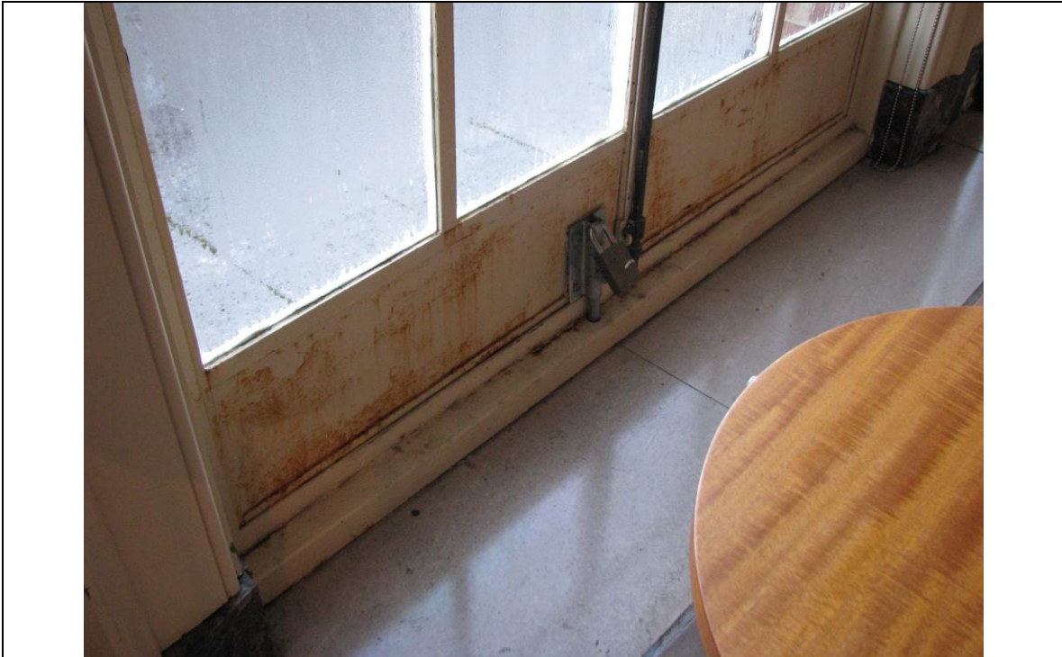
Figure 1.2.3-17: Rusty bottom rail, typical at West Terrace doors. Photograph by John Milner Architects, November 2012.
