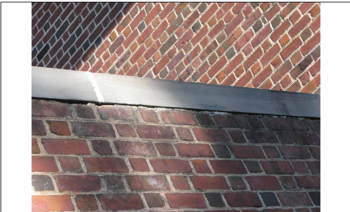
Figure 1.2.3-6: Open joint below parapet coping at West Terrace. Photograph by John Milner Architects, November 2012.
