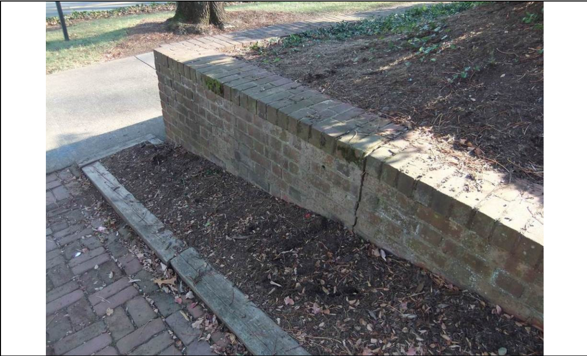
Figure 1.2.4.1-27: Localized brick-masonry vertical cracking at the retaining wall perpendicular to Rugby Road on the north side of the site. Photograph by Robert Silman Associates, November 2012.
