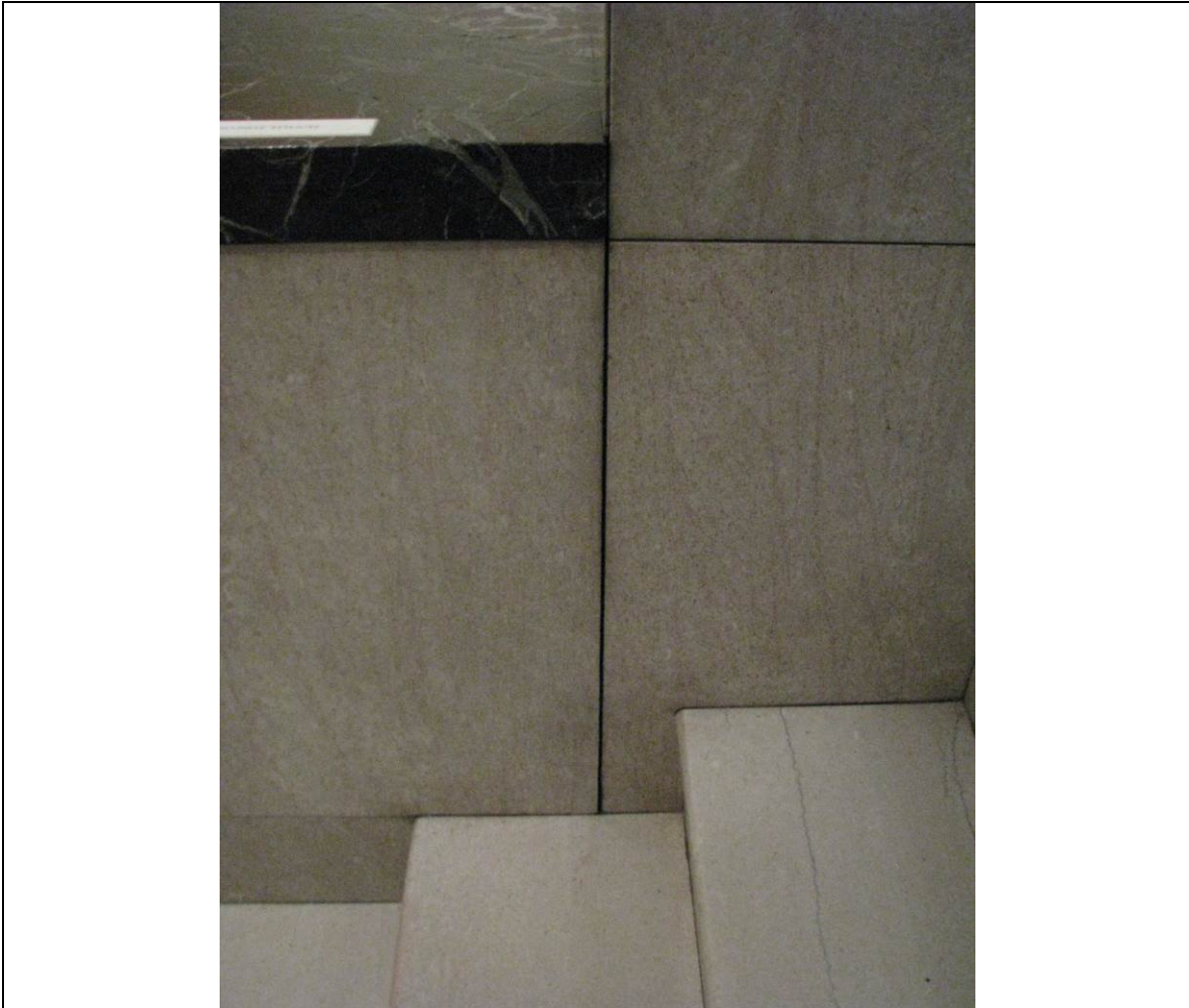
Figure 1.2.3-35: Open grout joints in marble panels at stair. Photograph by John Milner Architects, November 2012.
