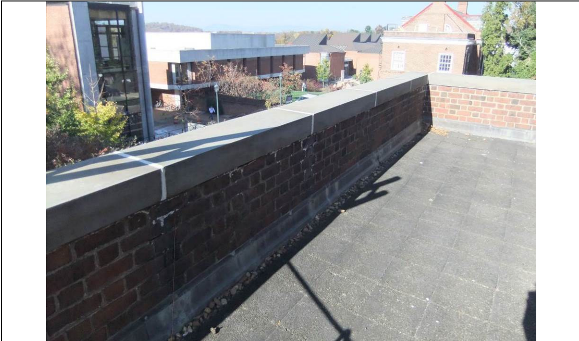
Figure 1.2.4.1-11: Parapet of West Terrace. Note: Biological growth, caulking of head joints, and loss of mortar at bed joints. Photograph by Robert Silman Associates, November 2012.
