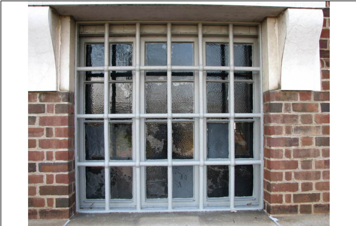
Figure 1.2.3-16: Cracked window panes. Photograph by John Milner Architects, November 2012.
