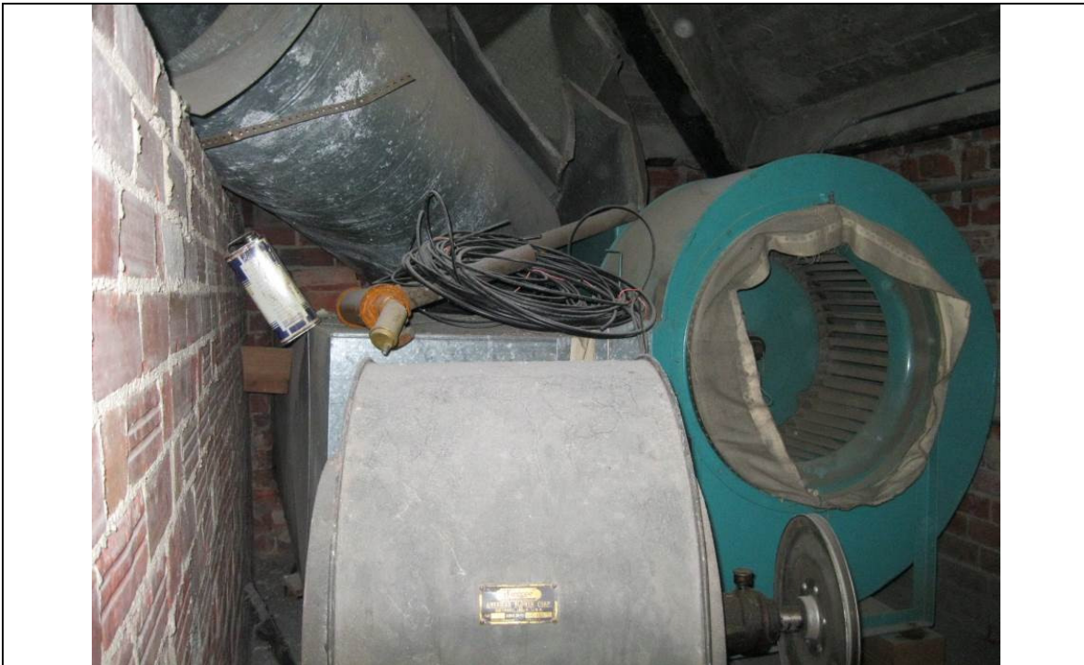
Figure 1.2.4.2-8: Abandoned exhaust fans in attic. Photograph by T. Newbold, December 2012.
