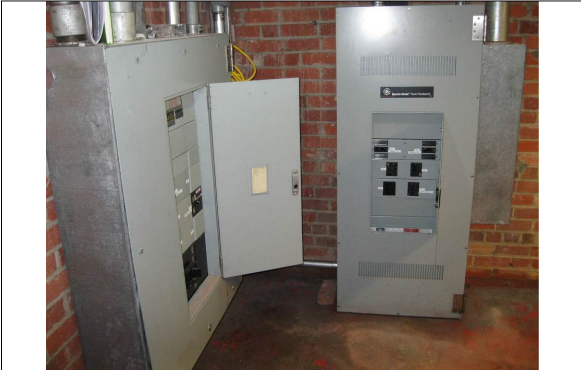
Figure 1.2.4.2-12: Distribution panels DP-1 and DP-2 in Annex elevator Modulation Error Ratio. Photograph by T. Newbold, December 2012.
