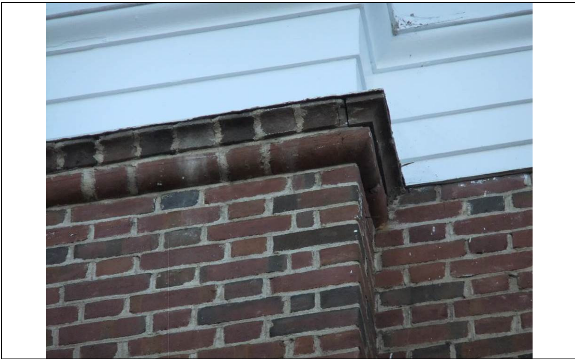
Figure 1.2.4.1-19: Localized loose brick and open mortar joints at top of pilasters. Photograph by Robert Silman Associates, November 2012.
