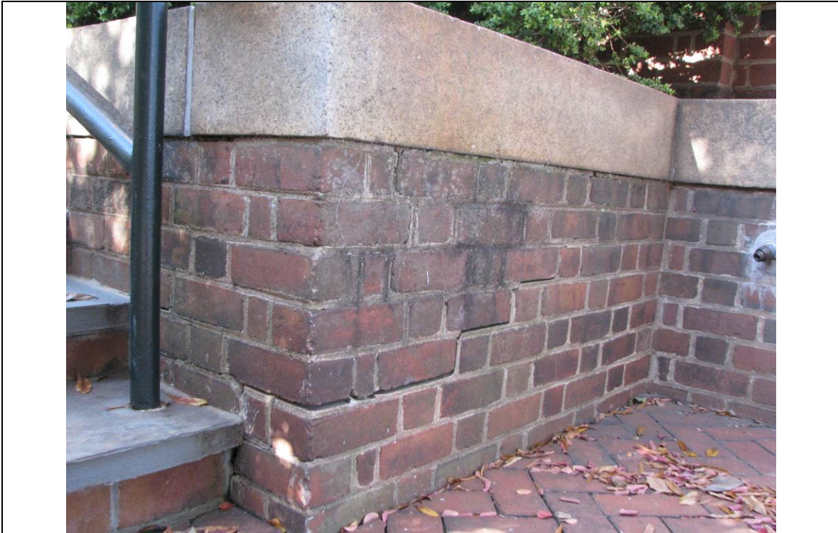
Figure 1.2.3-9: Distressed brickwork at south landscape wall. Photograph by John Milner Architects, November 2012.
