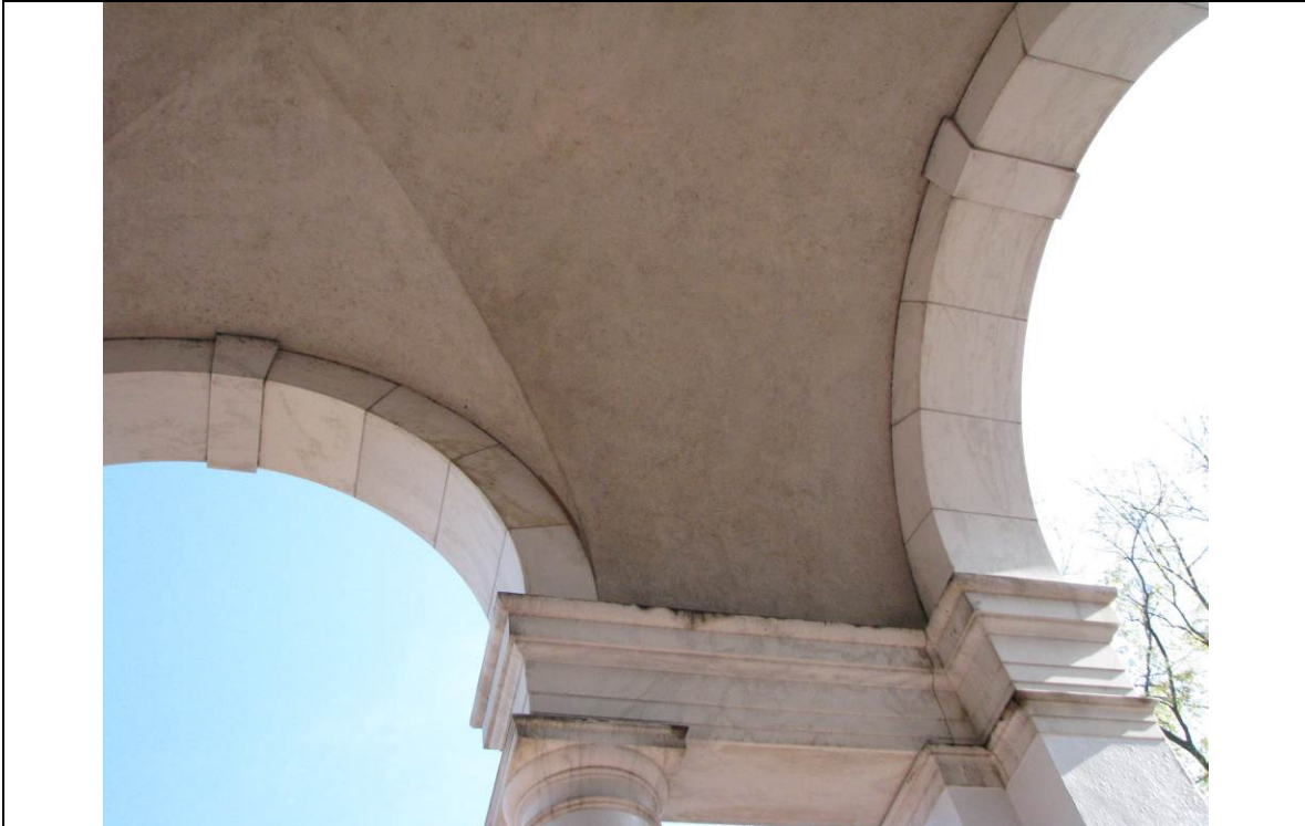
Figure 1.2.3-13: Soiling of Portico marble elements, typical. Photograph by John Milner Architects, November 2012.
