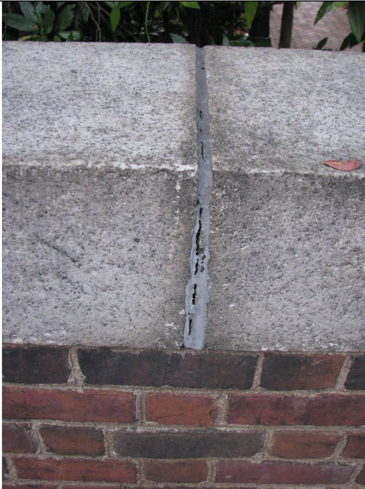
Figure 1.2.3-11: Failed sealant, typical at granite course. Photograph by John Milner Architects, November 2012.
