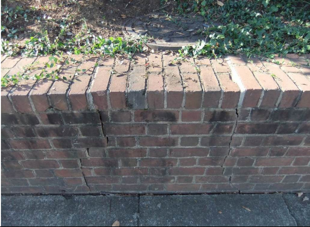
Figure 1.2.4.1-31: Vertical cracking in brick-masonry site wall locally at existing sanitary and water lines. Photograph by Robert Silman Associates, November 2012.
