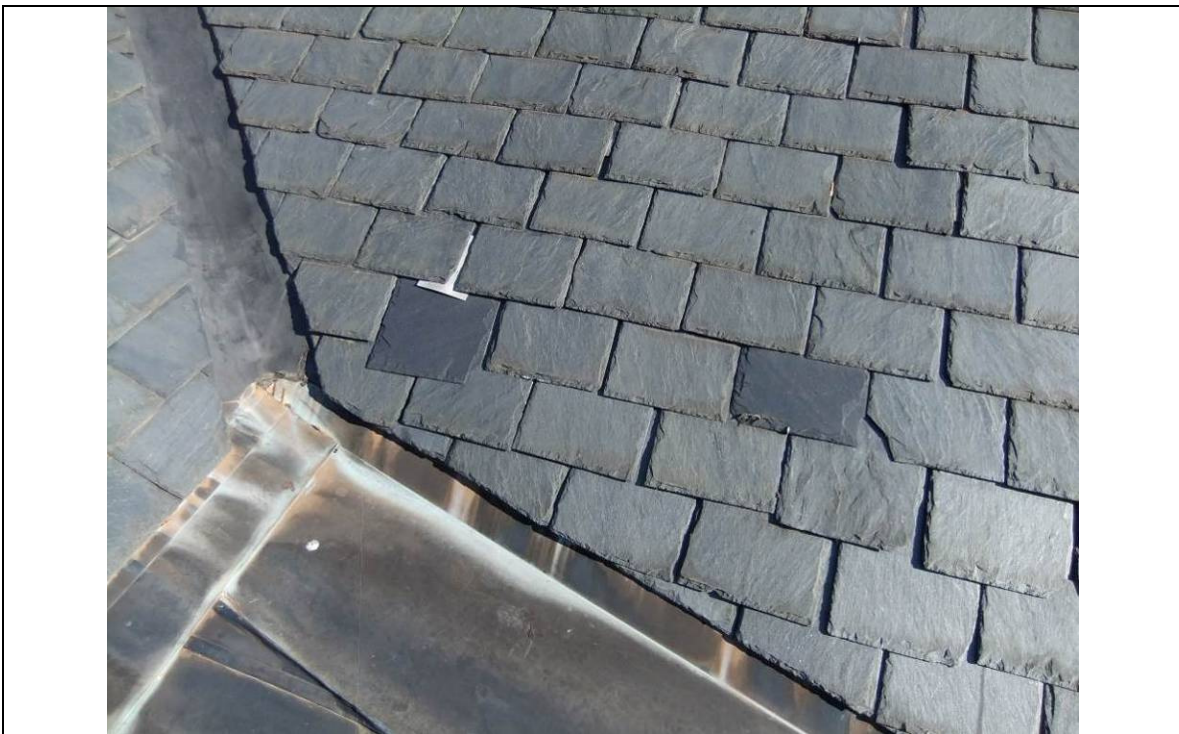
Figure 1.2.4.1-10: Localized slate deterioration at valley of roof. Photograph by Robert Silman Associates, November 2012.
