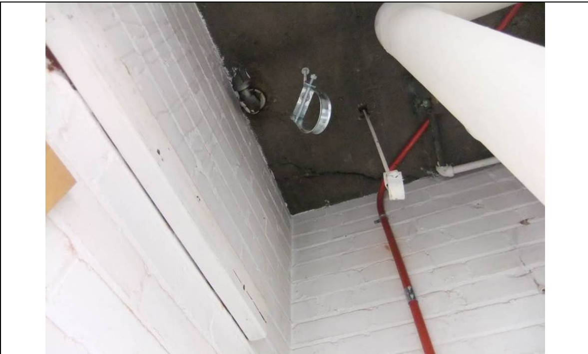
Figure 1.2.4.1-15: Crack in underside of first-floor slab in northeast mechanical room above trench access hatch. Photograph by Robert Silman Associates, November 2012.
