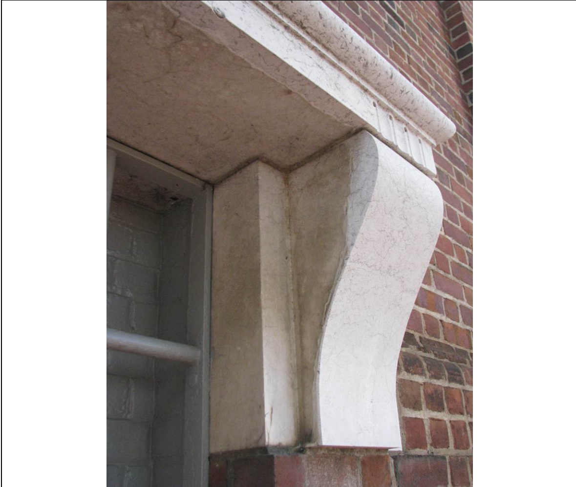
Figure 1.2.3-12: Aggressively and incompletely cleaned marble window sill and bracket, typical at East facade. Photograph by John Milner Architects, November 2012.
