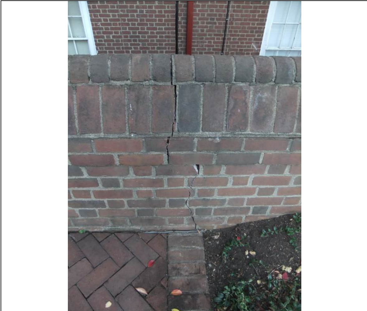
Figure 1.2.4.1-26: Localized brick-masonry vertical cracking at retaining wall along northern boundary of site. Photograph by Robert Silman Associates, November 2012.
