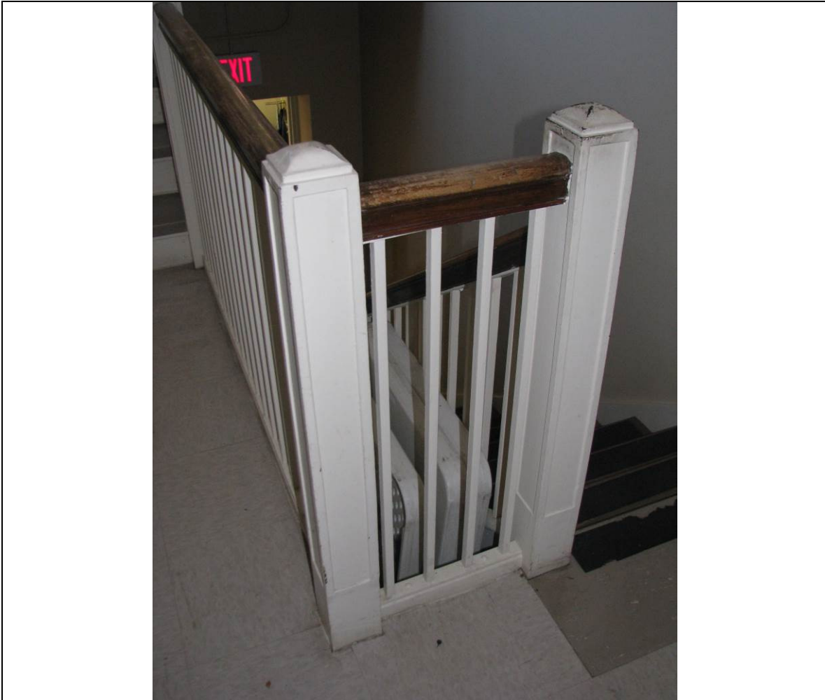
Figure 1.2.3-36: Worn railings and newels at secondary staircase. Photograph by John Milner Architects, November 2012.
