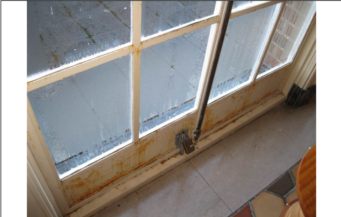
Figure 1.2.4.2-1: Single-glazed door on second floor with condensation. Photograph by T. Newbold, December 2012.
