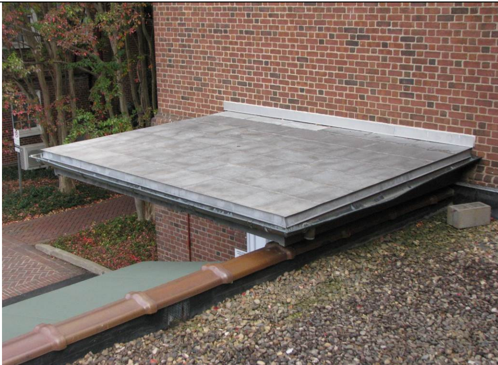
Figure 1.2.3-30: Deformed gutter at West canopy. Photograph by John Milner Architects, November 2012.
