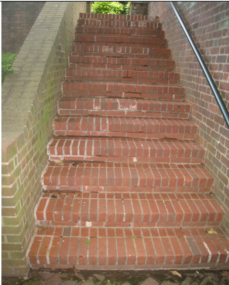
Figure 1.2.1-8: Water infiltration is evident as well as a partial bright mortar repointing at the brick steps at the west end of the South Garden. Photograph by Heritage Landscapes, June 2012.
