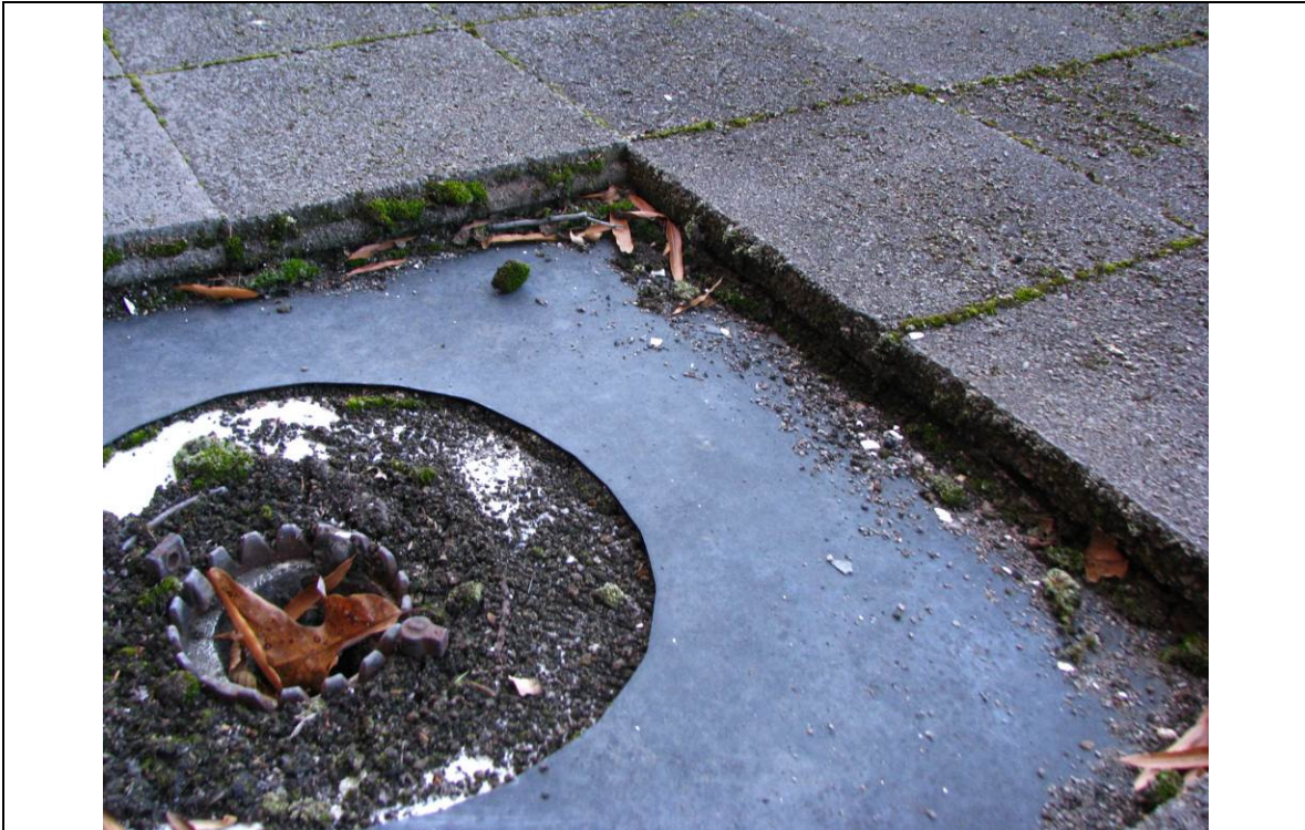
Figure 1.2.3-23: Unprotected terrace drain. Photograph by John Milner Architects, November 2012.
