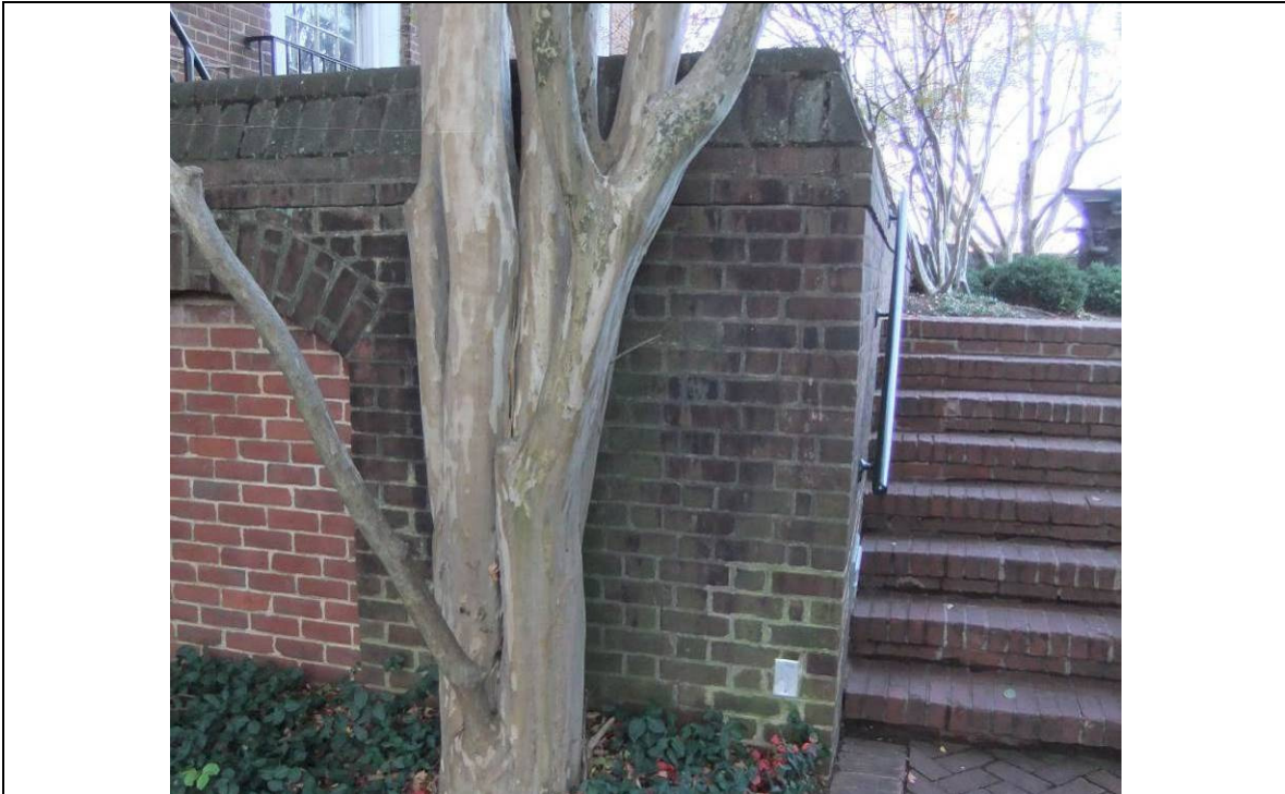
Figure 1.2.4.1-24: Existing brick-masonry retaining wall at northwest corner of site exhibiting localized vertical cracking due to proximity of tree-root and underlying root-system encroachment. Photograph by Robert Silman Associates, November 2012.
