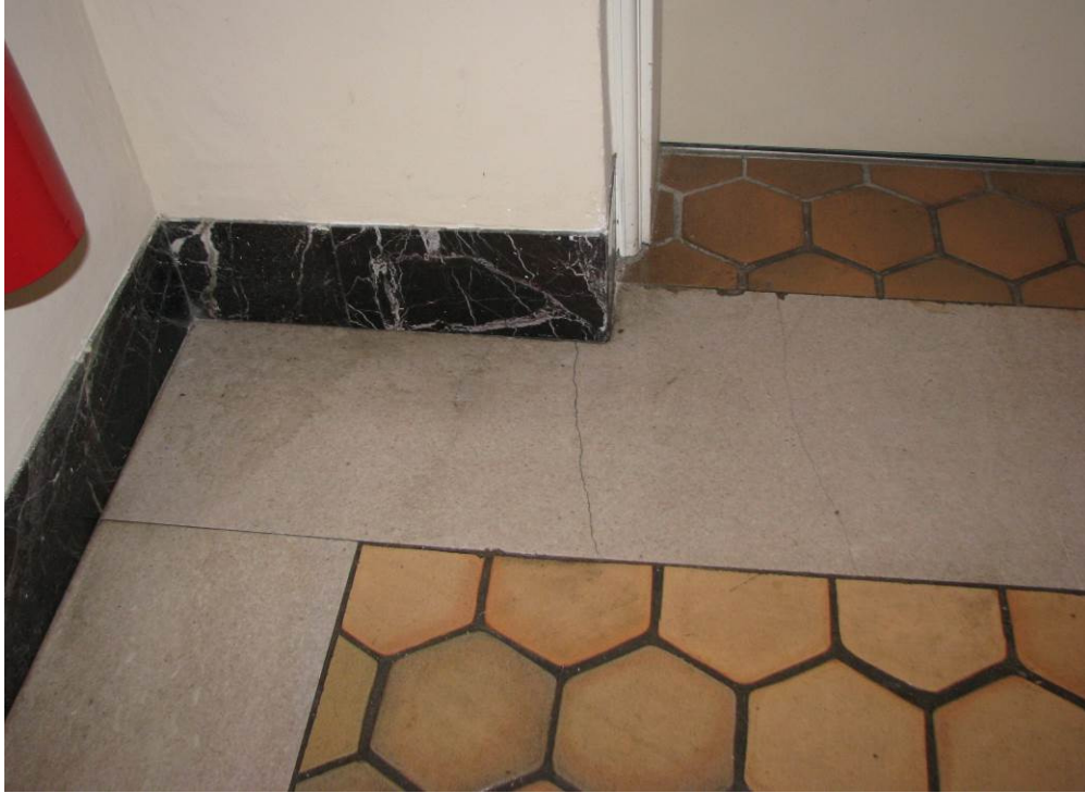
Figure 1.2.3-32: Hairline cracks in Tennessee Tavarnelle marble border. Photograph by John Milner Architects, November 2012.
