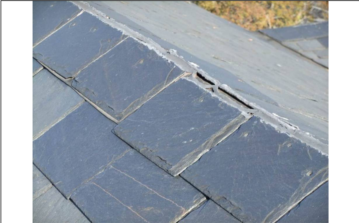
Figure 1.2.4.1-9: Localized slate deterioration at apex of roof. Photograph by Robert Silman Associates, November 2012.
