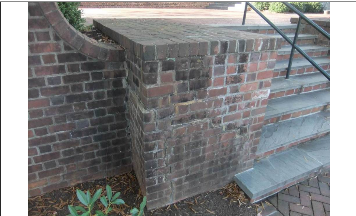
Figure 1.2.4.1-28: Brick-masonry cracking and displacement of pier abutment due to retaining-wall movement. Photograph by Robert Silman Associates, November 2012.
