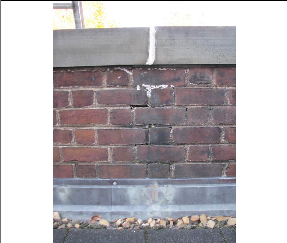
Figure 1.2.3-2: Open joints at West Terrace parapet, below inappropriately sealed coping joint. Photograph by John Milner Architects, November 2012.
