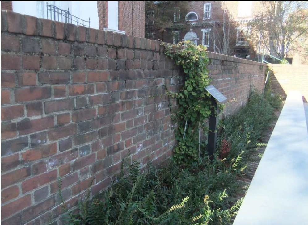
Figure 1.2.4.1-32: Biological growth and efflorescence in brick-masonry retaining wall. Photograph by Robert Silman Associates, November 2012.
