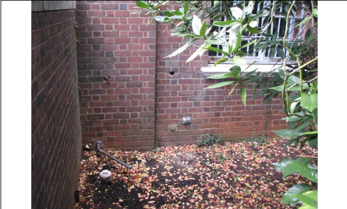
Figure 1.2.3-8: Abandoned open penetrations at northeast corner. Photograph by John Milner Architects, November 2012.
