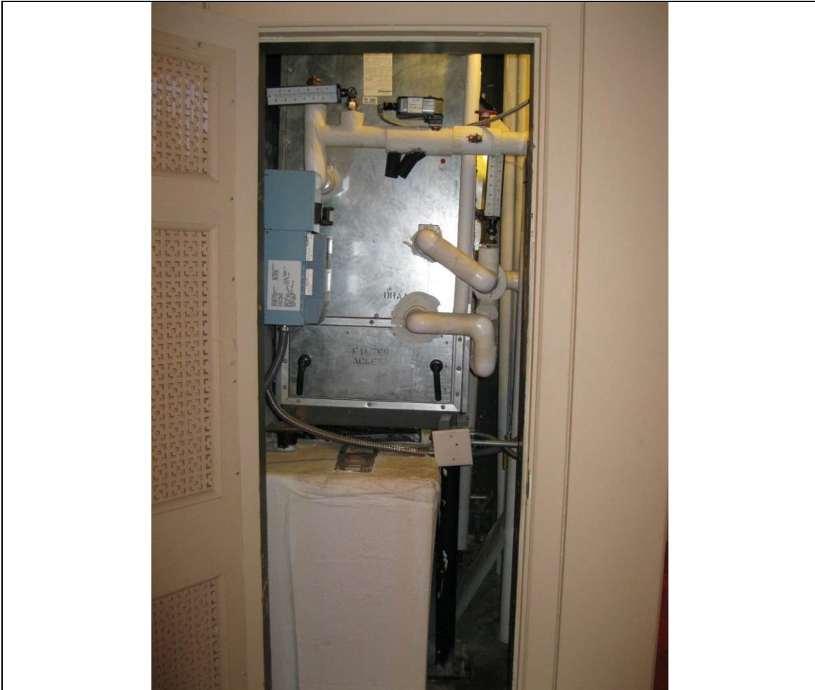
Figure 1.2.4.2-6: Air handler AHU-6 in second-floor closet. Photograph by T. Newbold, December 2012.
