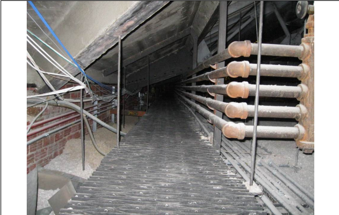
Figure 1.2.4.2-7: Abandoned skylight heating system in attic. Photograph by T. Newbold, December 2012.
