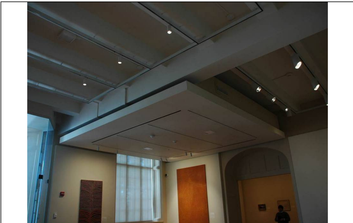
Figure 1.3.2-25: Non-character-defining air-distribution system suspended beneath Exhibition Lobby ceiling. Photograph by John Milner Architects, November 2012.
