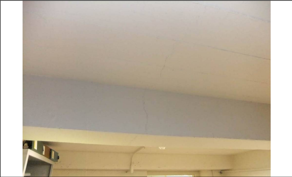
Figure 1.2.4.1-14: Crack in underside of first-floor slab and beam encasement in existing storage room adjacent to elevator. Photograph by Robert Silman Associates, November 2012.
