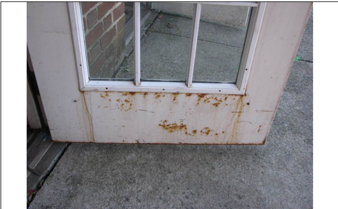
Figure 1.2.3-18: Rusty bottom rail at Annex door. Photograph by John Milner Architects, November 2012.
