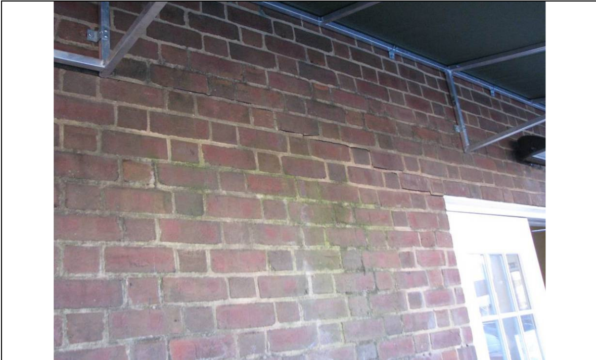
Figure 1.2.3-7: Running crack at Annex door head. Photograph by John Milner Architects, November 2012.
