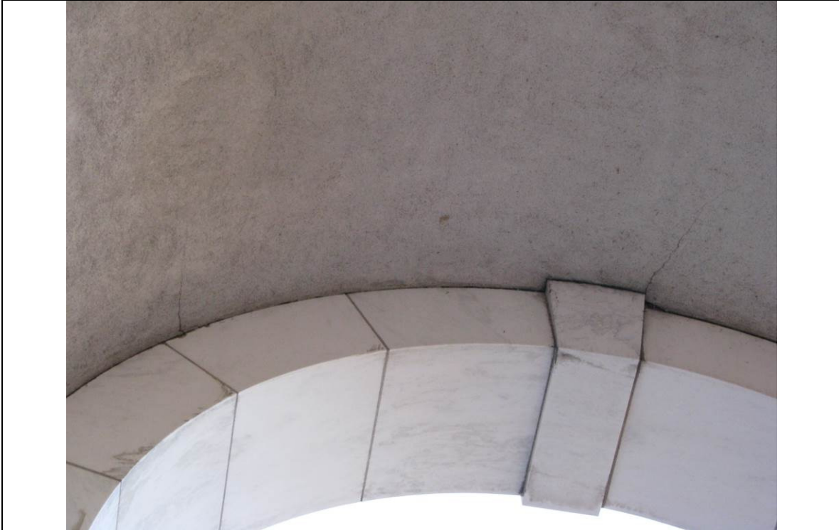
Figure 1.2.3-14: Hairline cracks at perimeter of Portico ceiling. Photograph by John Milner Architects, November 2012.
