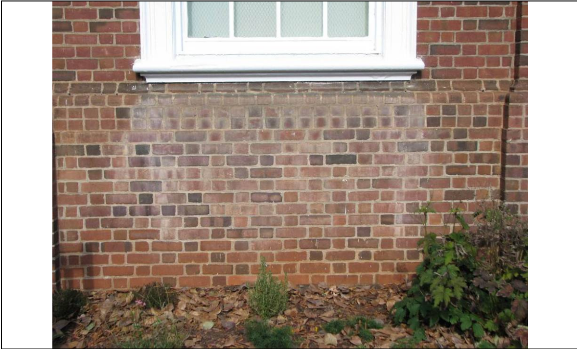
Figure 1.2.3-3: Stained brickwork, typical below windows. Photograph by John Milner Architects, November 2012.
