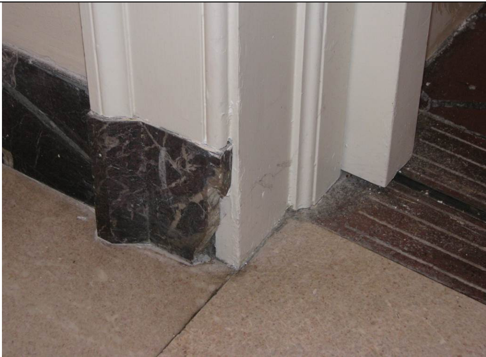
Figure 1.2.3-33: Broken Levanto marble wall base. Photograph by John Milner Architects, November 2012.
