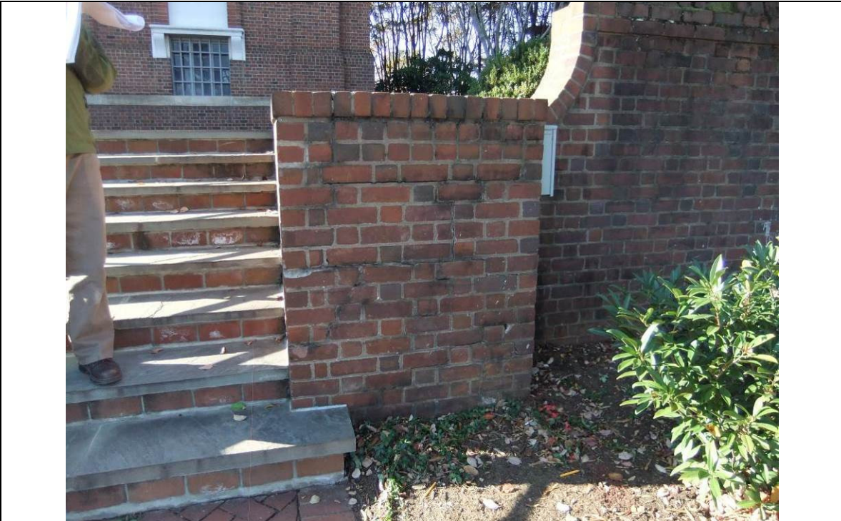
Figure 1.2.4.1-29: Horizontal cracking and displacement of brick at pier abutment due to retaining wall movement. Photograph by Robert Silman Associates, November 2012.
