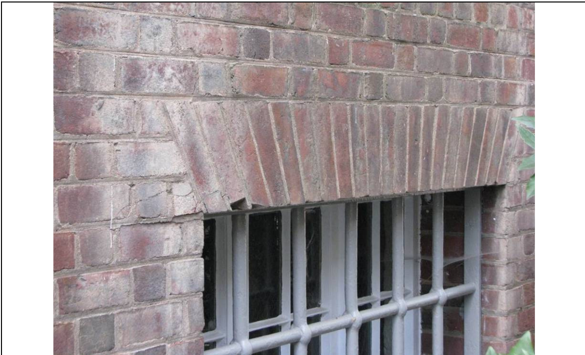
Figure 1.2.3-5: Distressed brickwork at window head, common at West and North facade basement openings. Photograph by John Milner Architects, November 2012.
