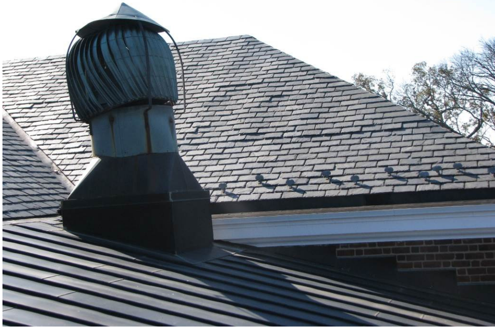
Figure 1.2.3-20: Damaged ventilator. Undulating roof surface (typical) visible beyond. Photograph by John Milner Architects, November 2012.
