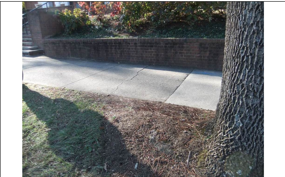
Figure 1.2.4.1-30: Cracking and heaving of concrete sidewalk slab due to tree-root encroachment. Photograph by Robert Silman Associates, November 2012.
