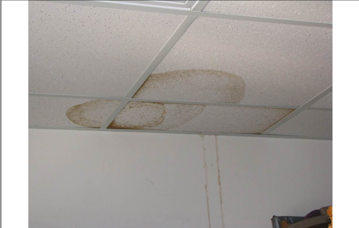
Figure 1.2.3-25: Water stains below southwest addition roof. Photograph by John Milner Architects, November 2012.
