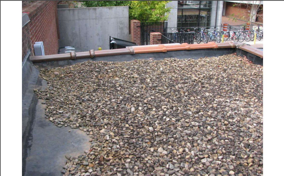
Figure 1.2.3-26: Sprung membrane and inappropriate coping patch at roof of Annex. Photograph by John Milner Architects, November 2012.
