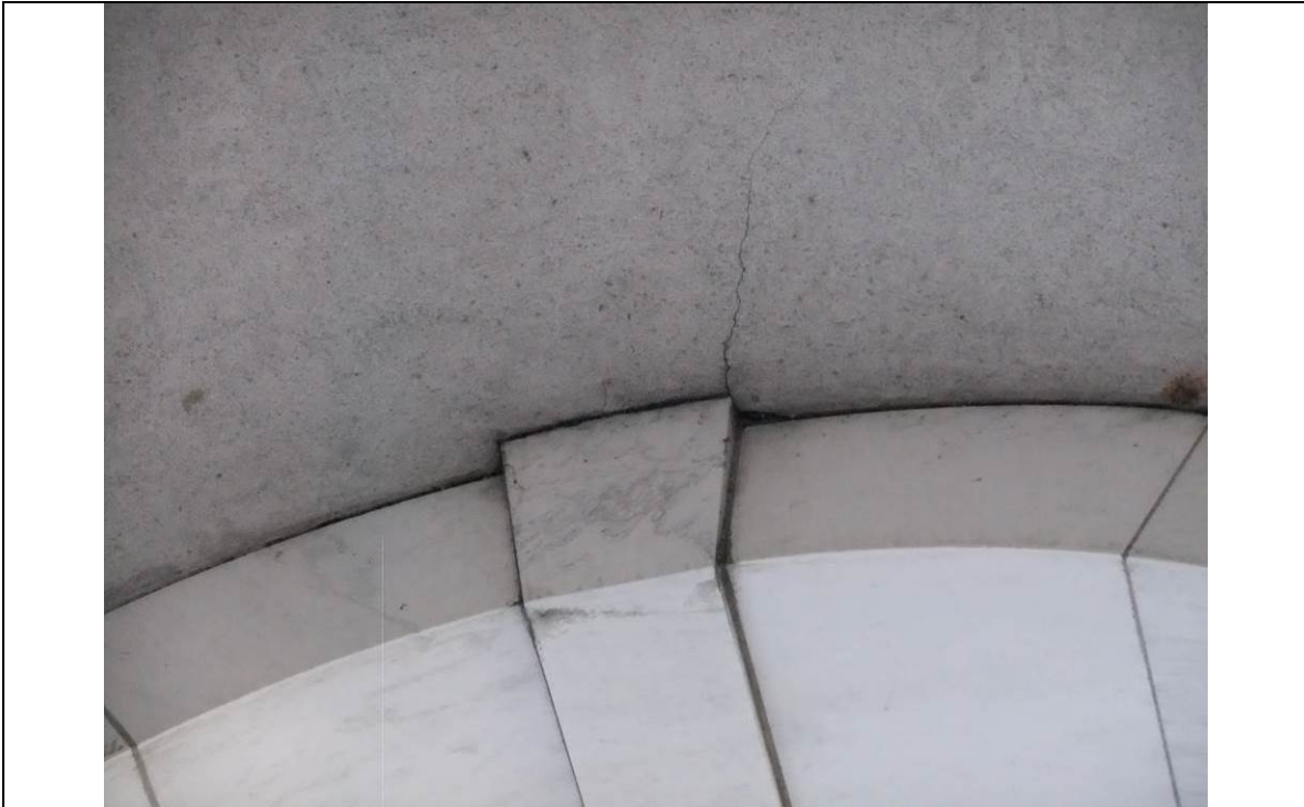
Figure 1.2.4.1-17: Localized cracking at top of hung stucco ceiling at east Portico. Photograph by Robert Silman Associates, November 2012.
