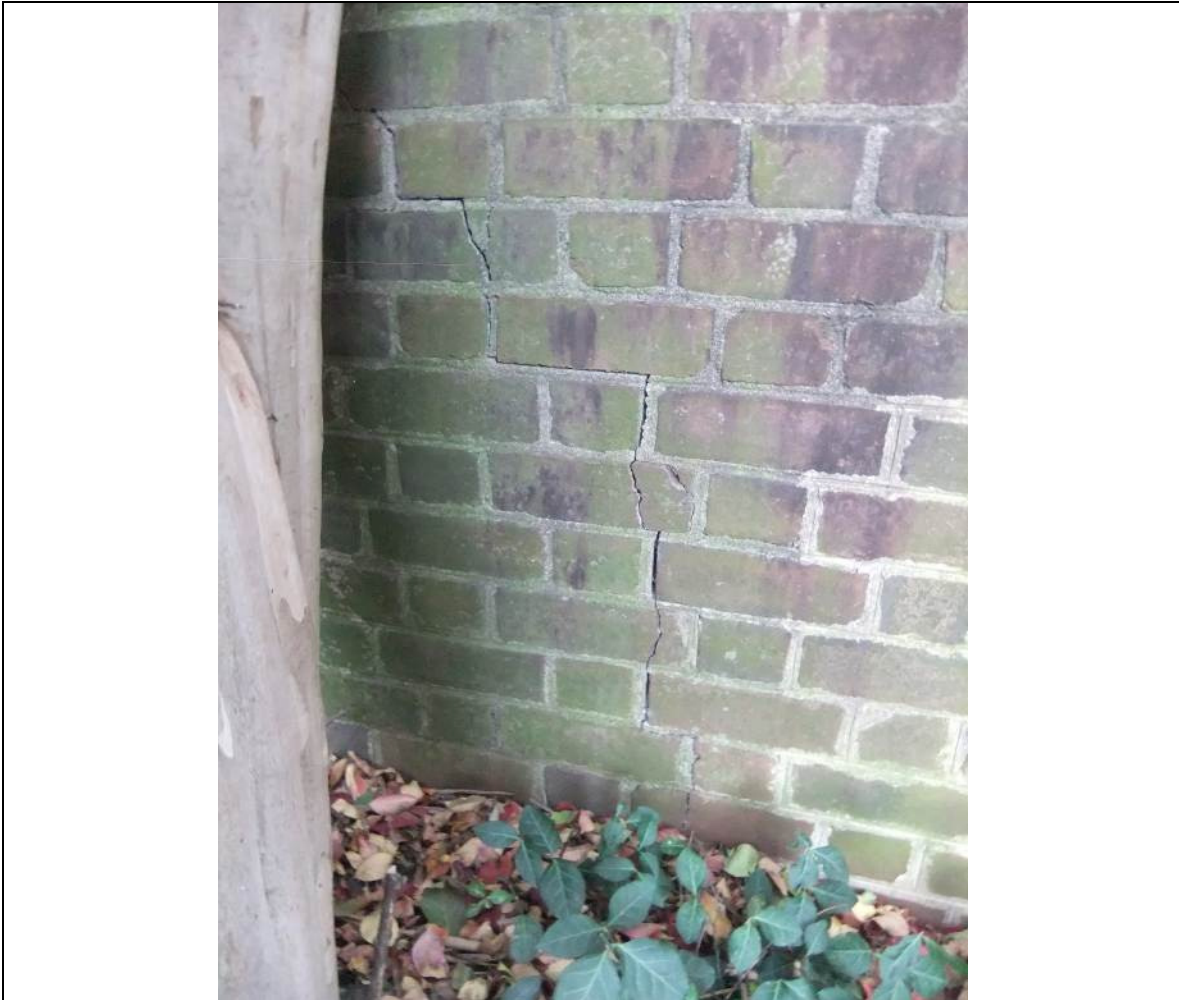
Figure 1.2.4.1-25: Existing brick-masonry retaining wall at northwest corner of site exhibiting localized vertical cracking due to proximity of tree-root and underlying root-system encroachment. Photograph by Robert Silman Associates, November 2012.
