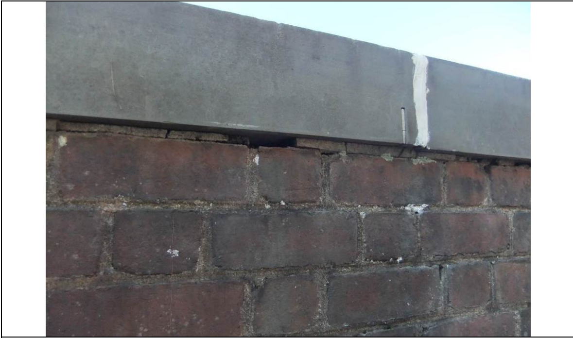
Figure 1.2.4.1-12: Parapet of West Terrace. Note: Biological growth, caulking of head joints, and loss of mortar at bed joints. Photograph by Robert Silman Associates, November 2012.
