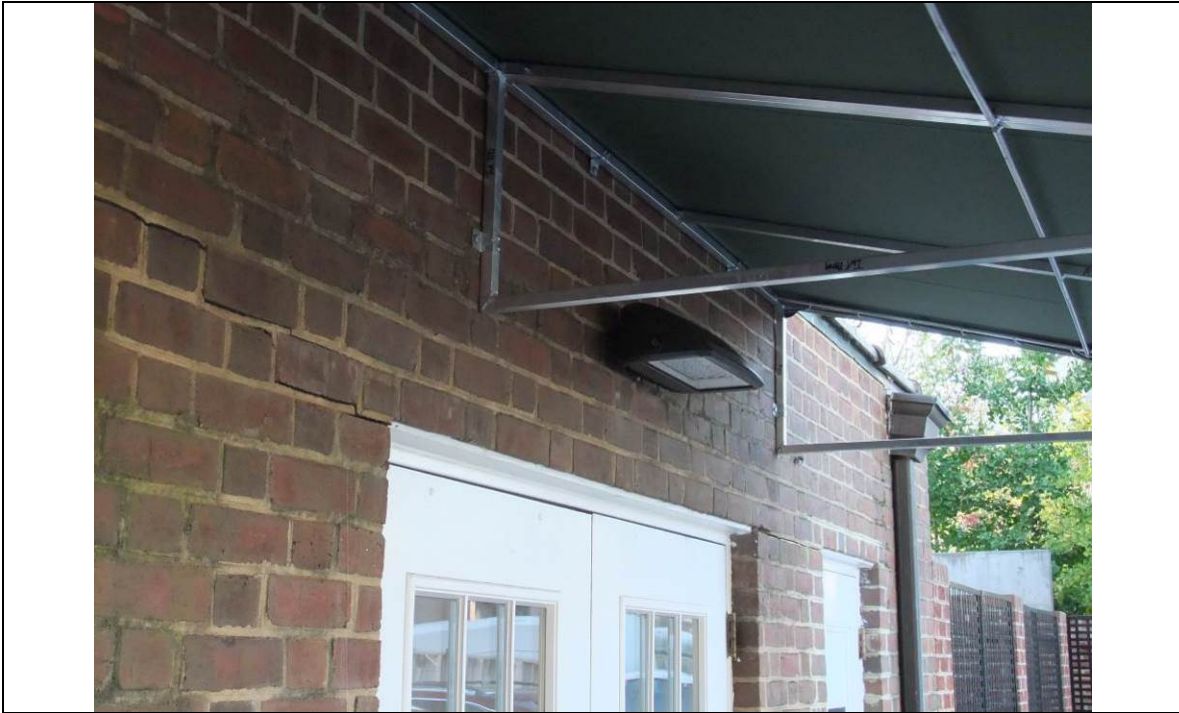
Figure 1.2.4.1-22: Horizontal cracking of brick masonry above wall penetrations (along single-story addition at northwest corner) due to rust jacking of steel lintels. Photograph by Robert Silman Associates, November 2012.
