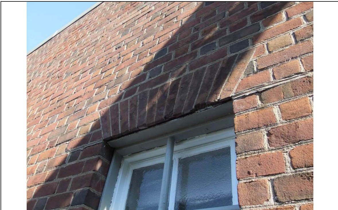
Figure 1.2.4.1-21: Deterioration of brick flat (jack) arch due to rust jacking of steel lintels along West elevation. Photograph by Robert Silman Associates, November 2012.
