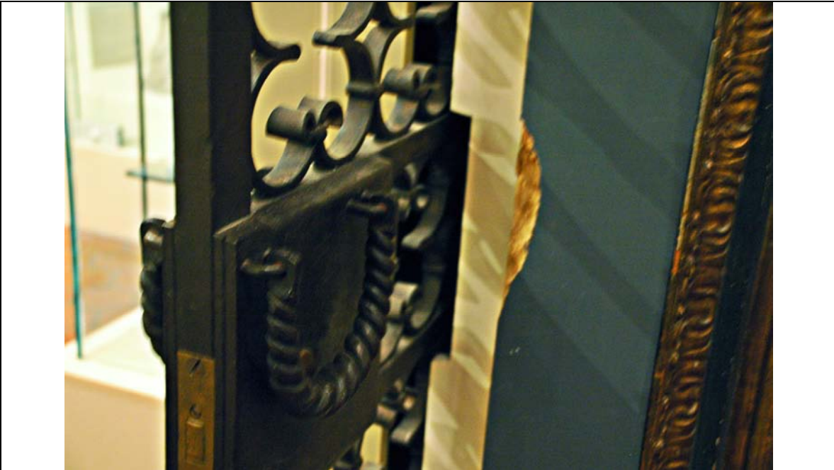
Figure 1.2.3-37: Damaged jamb at doorway to second-floor southwest gallery. Photograph by John Milner Architects, November 2012.
