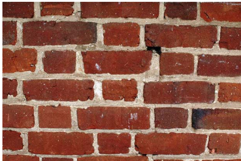
Mortar is an extremely soft lime mortar with frequent voids and cracks.
