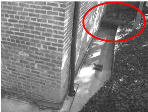
Underground conduits from IT closet into campus steam tunnel
