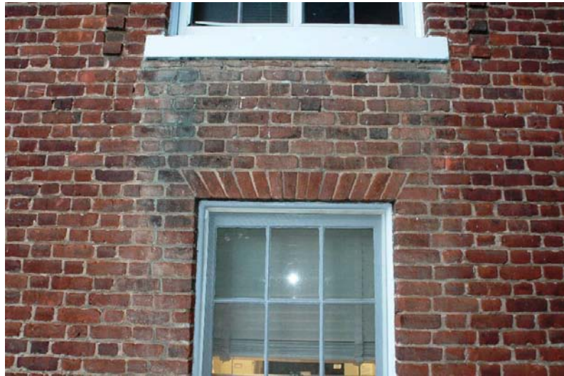
Typical staining beneath the windows.
