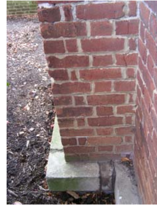
Photo 11: Cracking at east chimney
