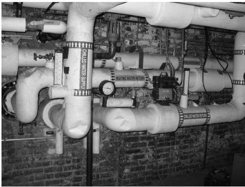
CHW and MTHW mains in mechanical room
