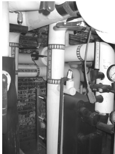
Heat exchanger in mechanical room
