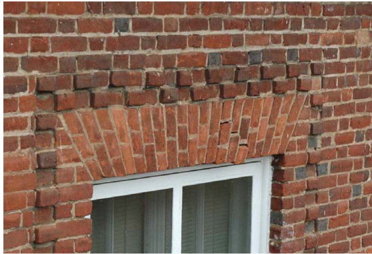
Rusticated artistic brick surrounds are typical at all principal windows. Note minor displacement of brick voussoirs at jack arch.
