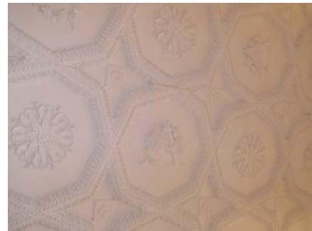
Photo 8: Cracking in decorative ceiling plaster
