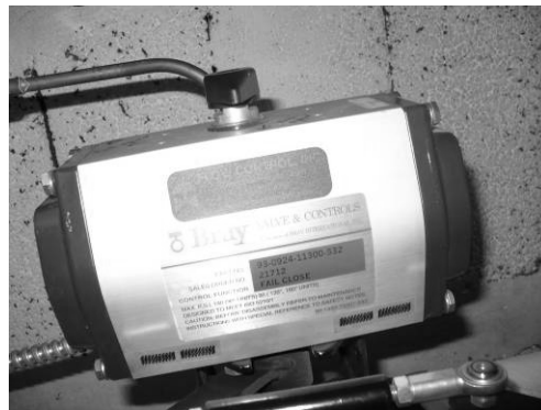
Pneumatic control in main mechanical vault
