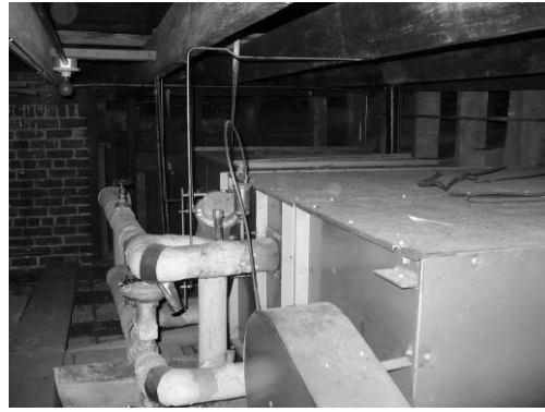
Air Handler above East Stairwell
