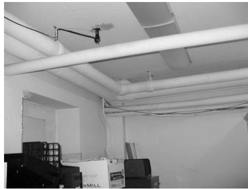
HVAC piping at ceiling of Basement
