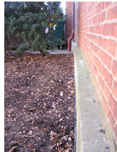
Photo 5: Exterior face of North wall – Area of inward bowing.
