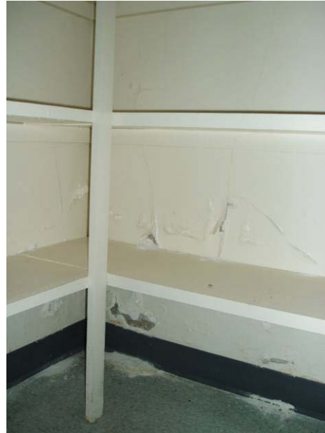
Plaster deterioration on closet walls below the exterior north stair
