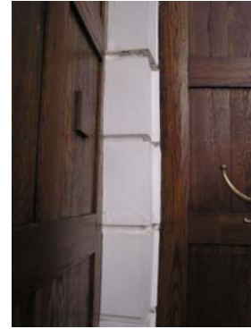
Photo 7: East Pilaster – Buckling wood paneling at inward-bowing wall
