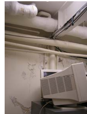
Photo 9: Water damage at Basement walls
