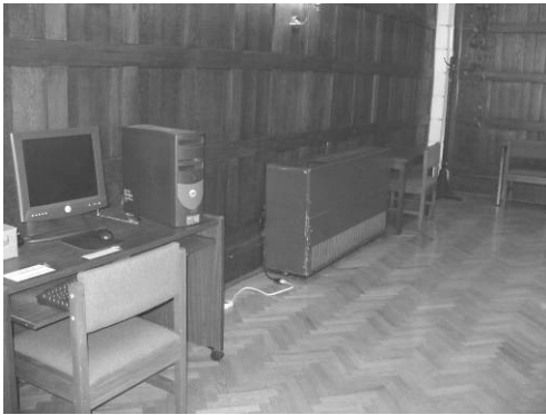
Unit ventilator in Main Hall
