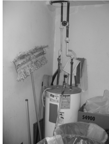
Water heater in Basement
