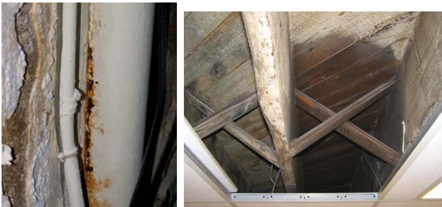
Figure 7: Rust at steel post fully developed thru wall thickness, also note plaster deterioration.
