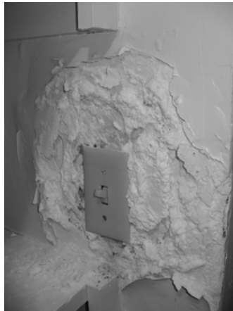
Wall switch in deteriorated wall
