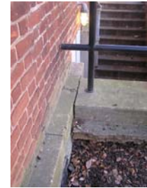
Photo 12: Separation at stairwell wall
