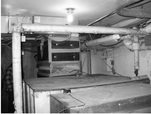
Air Handler in Basement
