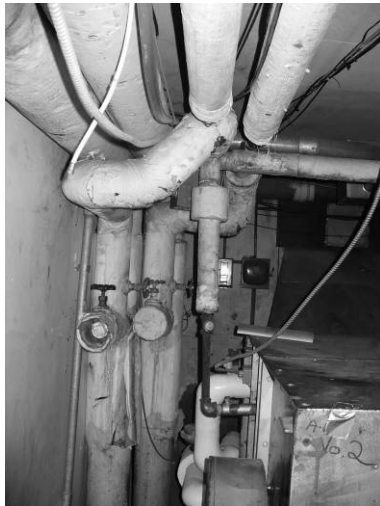
HVAC piping at Basement air handler
