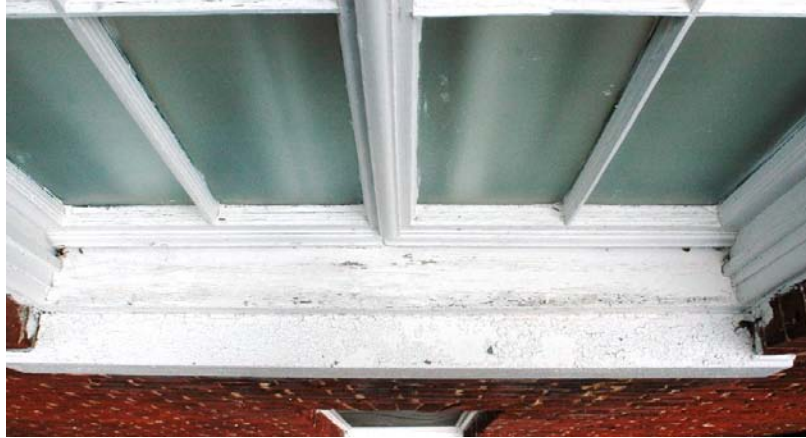
Window sills have a wood sill over a painted masonry sill (paint has typically failed).
