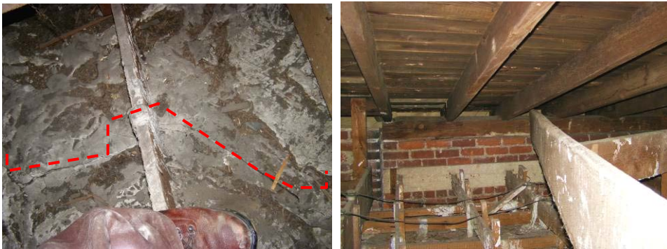
Figure 23: Crack as seen from attic space
