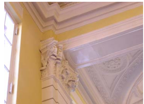
Photo 6: East Pilaster – Cracking at Capital
