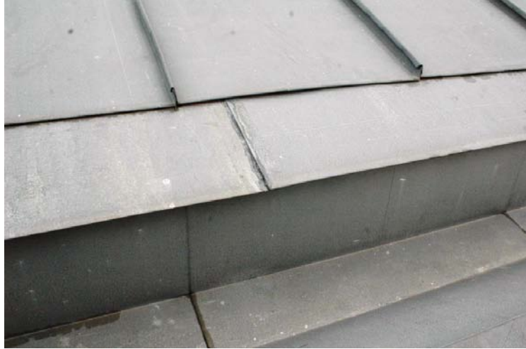
Soldered seams at the roof perimeter and in the gutter liner have failed.
