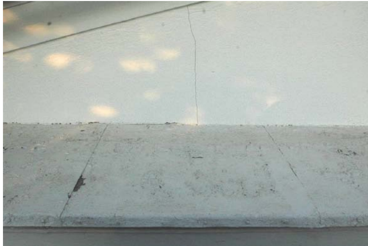
The pediment cornice flashing was not replaced during the 2001 re-roofing, has open seams, and is heavily over painted (note also crack in the stucco above).
