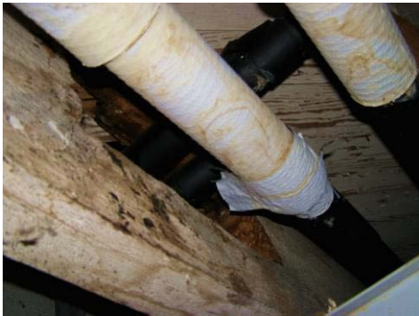
Figure 11: 1 st floor framing from women's bath. Note notch in joist.
