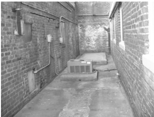
Outdoor condensing unit for IT closet
