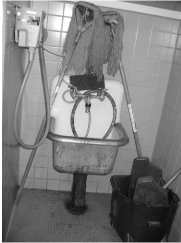
Service sink in Basement
