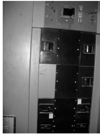
Outdated panel in Basement corridor
