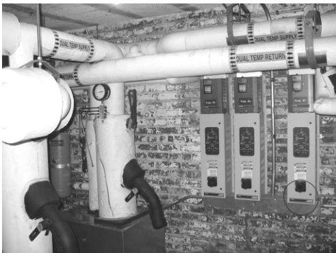
HW pump and variable frequency drives in mechanical room
