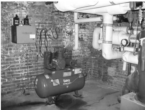
Air Compressor in main mechanical vault
